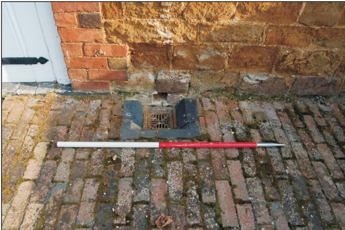
External drain originally serving the interior of the stable, looking north Plate 2
