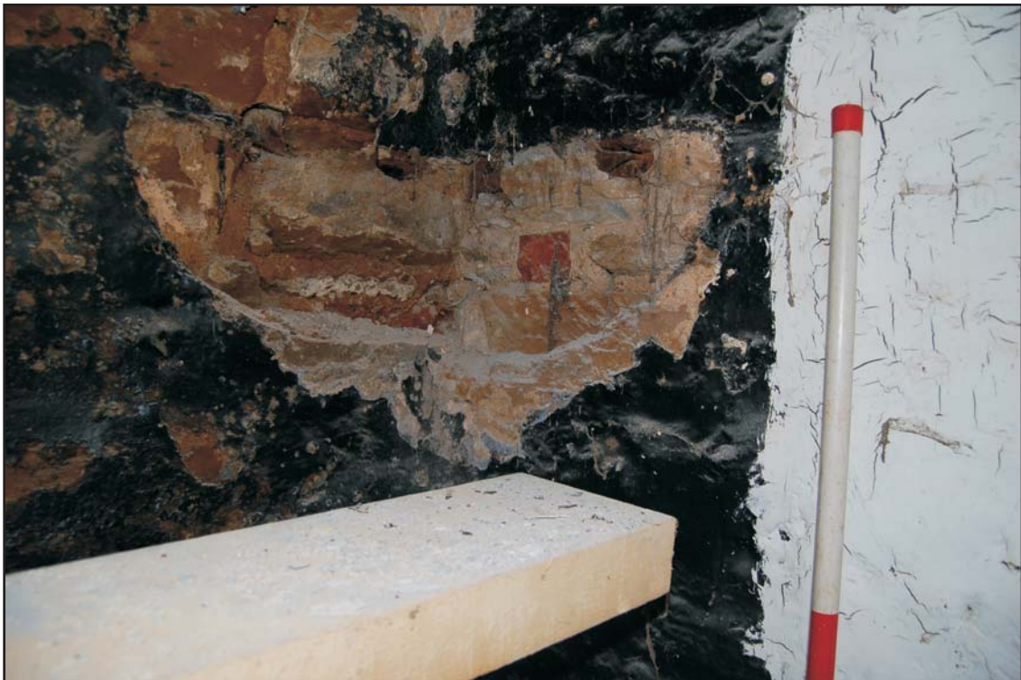
Scar showing the former location of the cast-iron corner trough in the north-east corner of the stables
