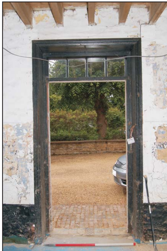
The stable door showing the boarded jambs and glazed overdoor panel, Plate 10 looking south
