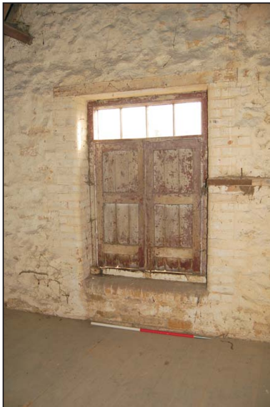
The hayloft door in the first floor east gable, looking east Plate 14
