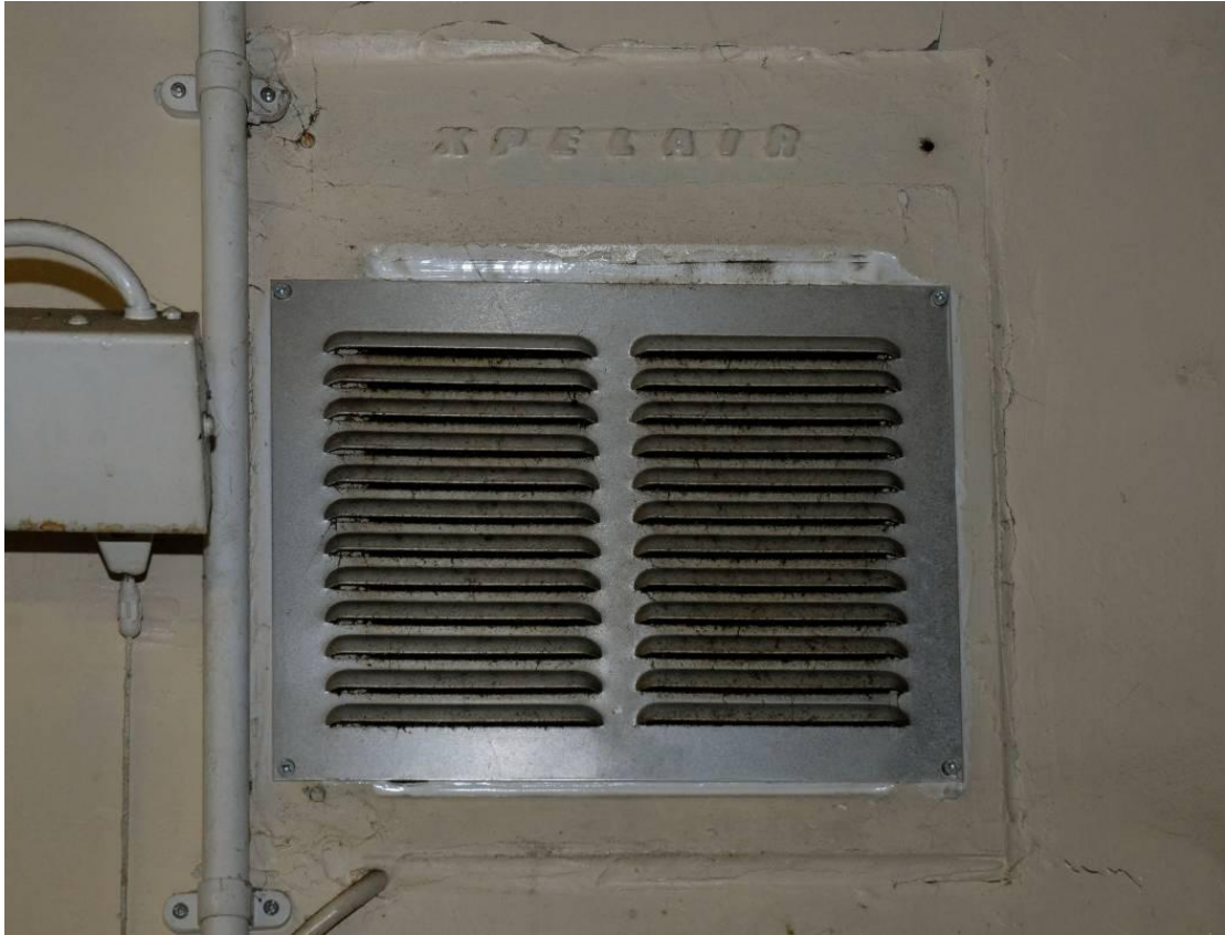
The original Xpelair fascia in the Kitchen Fig 13
