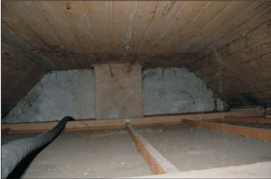
Room G11, roof space showing original matchboard ceiling and inserted modern ceiling, looking east
