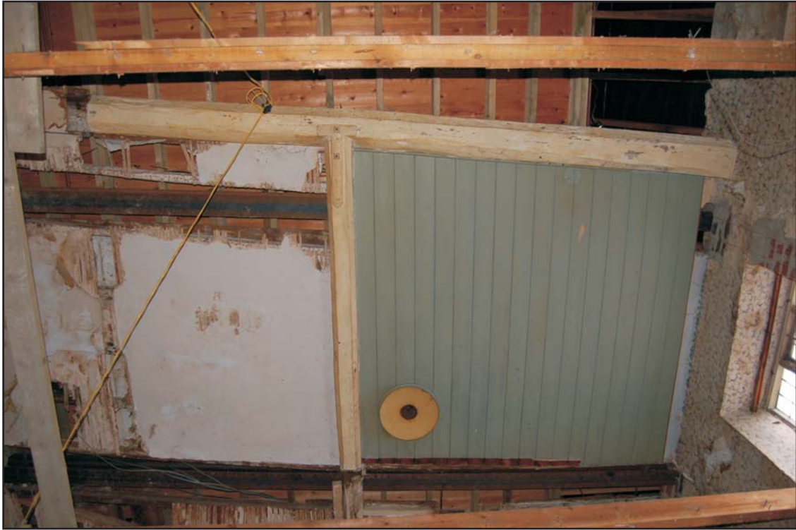
Room G5, looking up, showing ceiling to second floor with original oak beams and modern steels above
