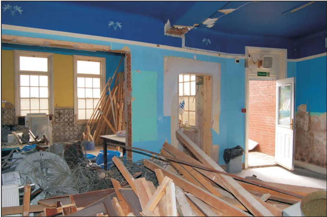
Room G7 (foreground) and Room G8 (left of photo), looking east Plate 18
