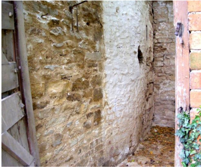
The east wall inside the tool shed; showing the whitewashed bulging rebuild Fig 23
