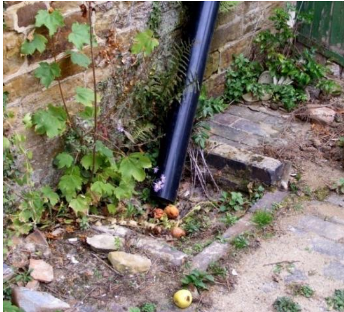
Plastic downpipe emptying into brick-lined drain outside Stable 2 Fig 17
