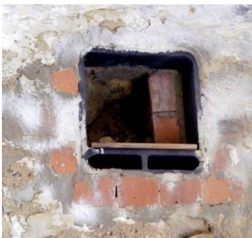
Stable 3, modern fitting Fig 48
