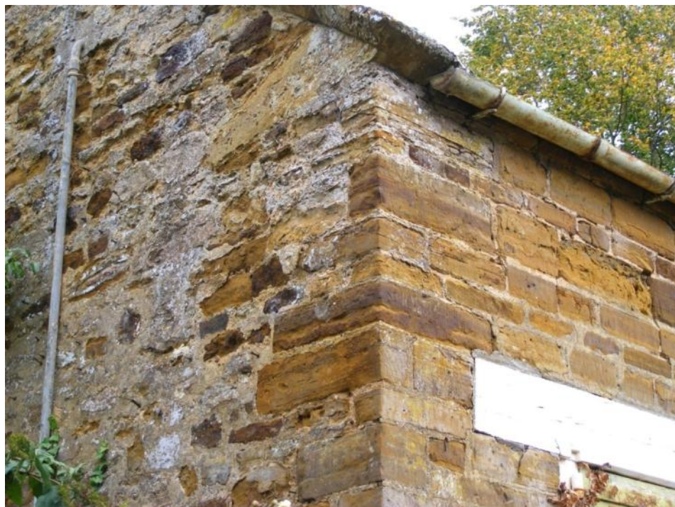
Detail of south elevation and gable end to show contrasting builds Fig 5
