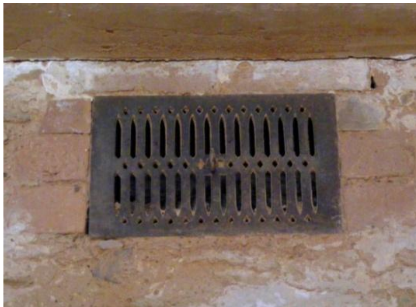
Stable 2, ventilator grille Fig 42
