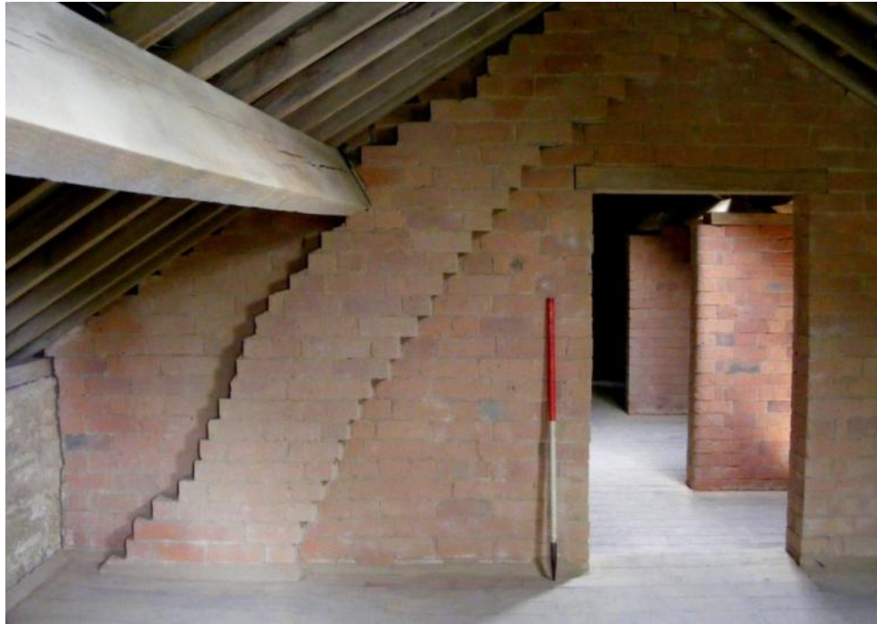
The hayloft, looking east, showing the chimney flue in the partition wall Fig 57
