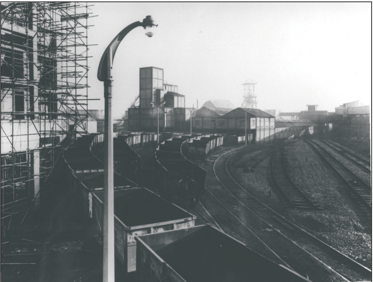
Coal preparation plant under construction, looking north-east. Undated. Copyright Leicestershire County Council Fig 10
