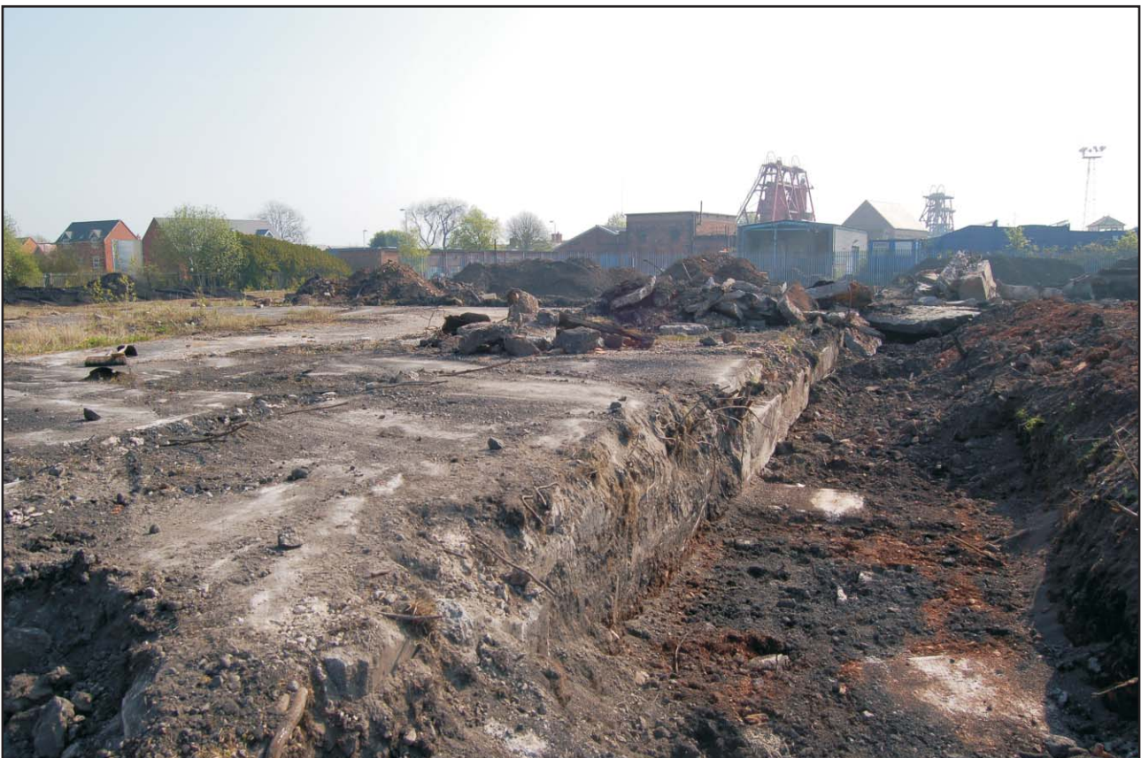
Concrete floor slabs to coal preparation plant building, looking north east Fig 16
