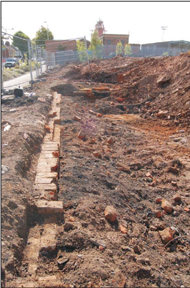
The street frontage foundations of the row of cottages, looking east Fig 19
