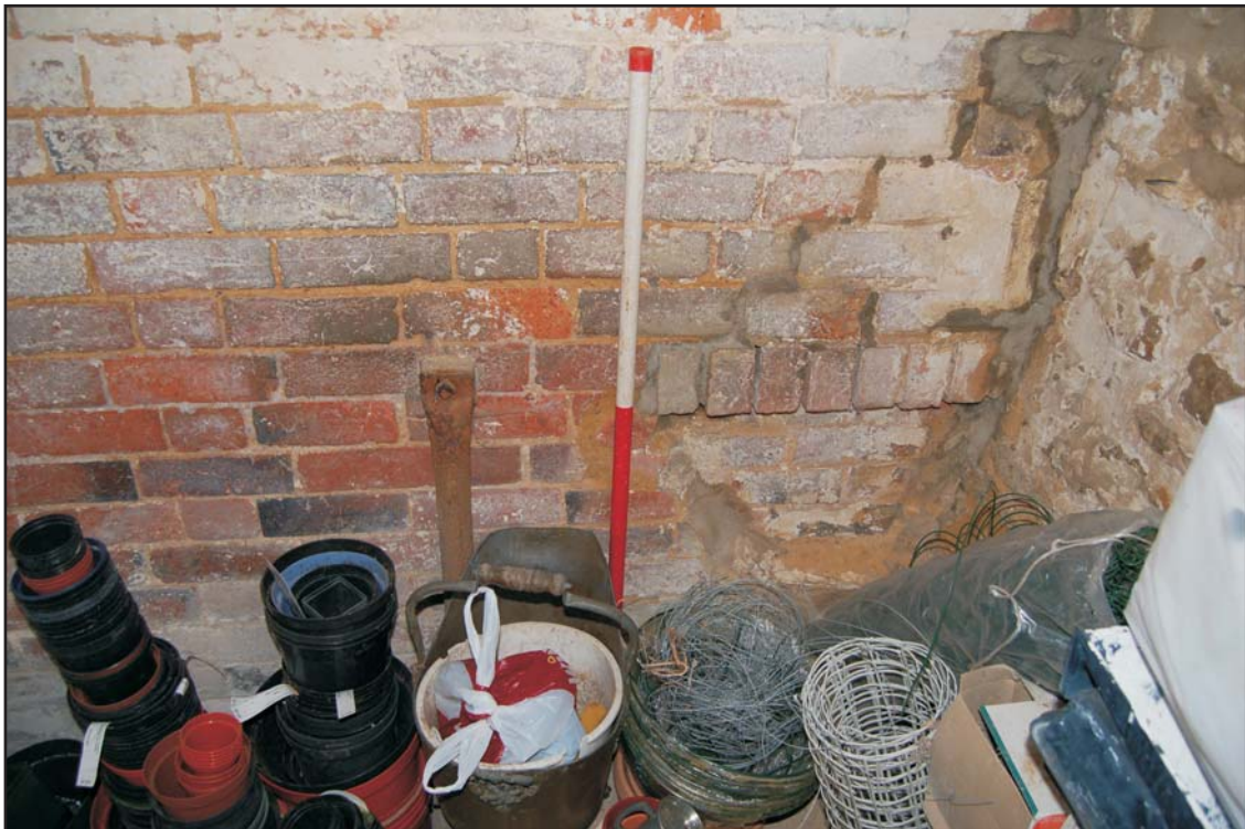
Recess indicating size and profile of former manger, east side of the dividing wall
