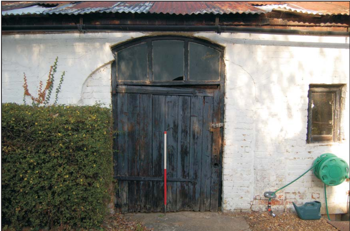
Arch 3 exterior and inserted timber door- note the chopped-out brickwork of the upper arch
