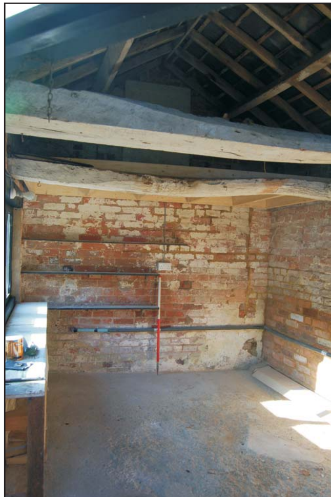
Store room, interior, looking west showing transverse beams for former hayloft floor Plate 13
