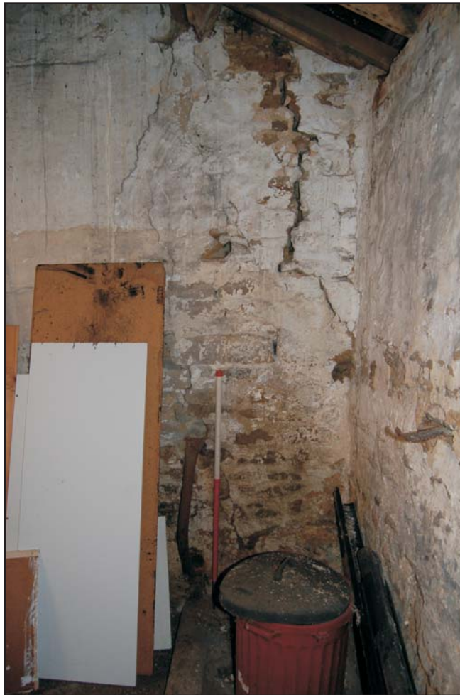
West wall interior elevation with empty sockets of former manger, east side of the dividing wall
