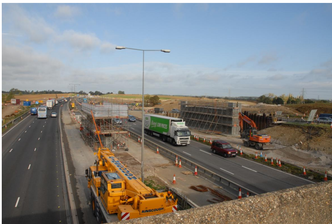
View from the M1 Junction 12 Overbridge looking north-west, showing the construction of the new bridge
