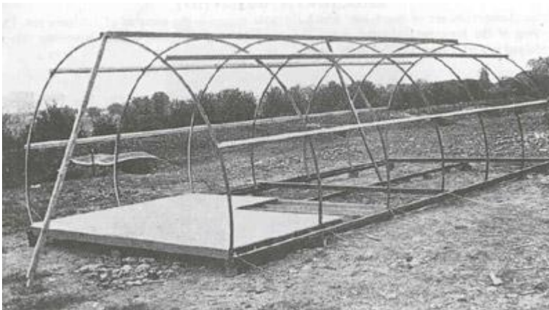
Wooden joists, to support the wooden floor panels, are screwed to the bearers Fig 4
