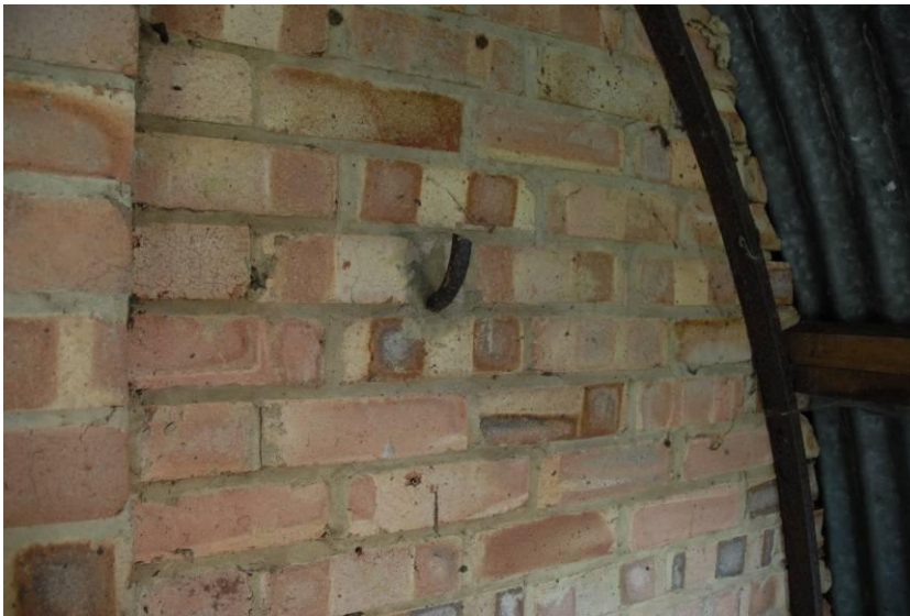
The inside of the front wall showing where the wiring came through from the junction box Fig 20
