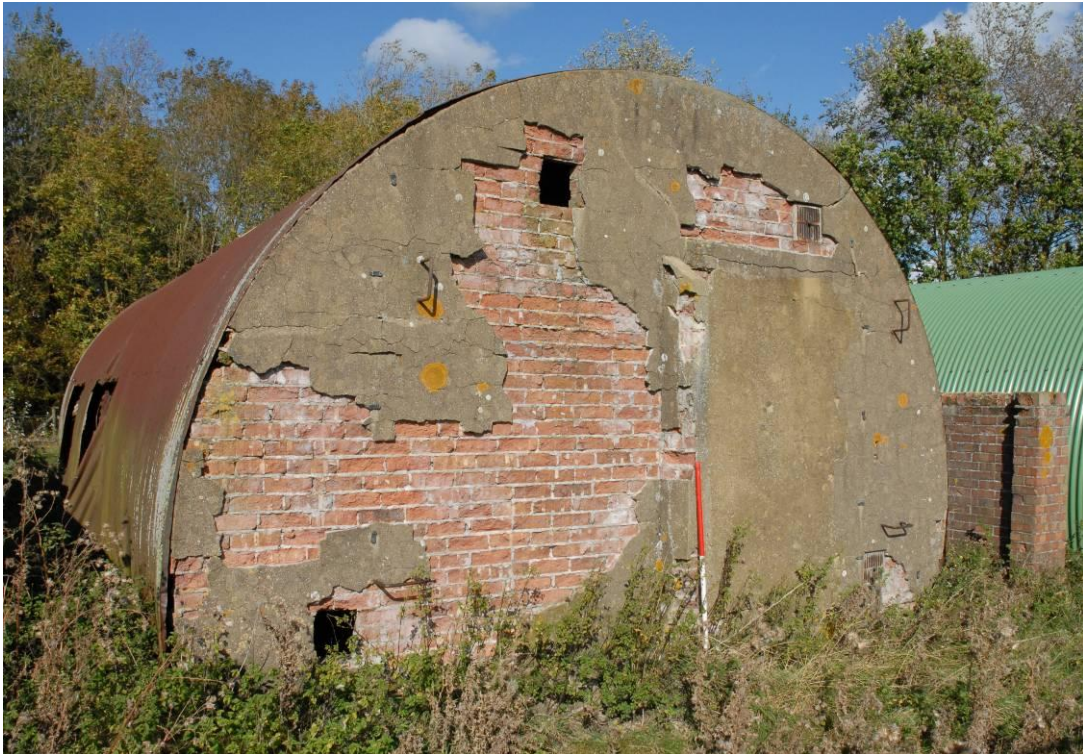
Back wall of Hut 141 showing concrete render over the blocked door, the vents and four iron rungs, looking north Fig 11
