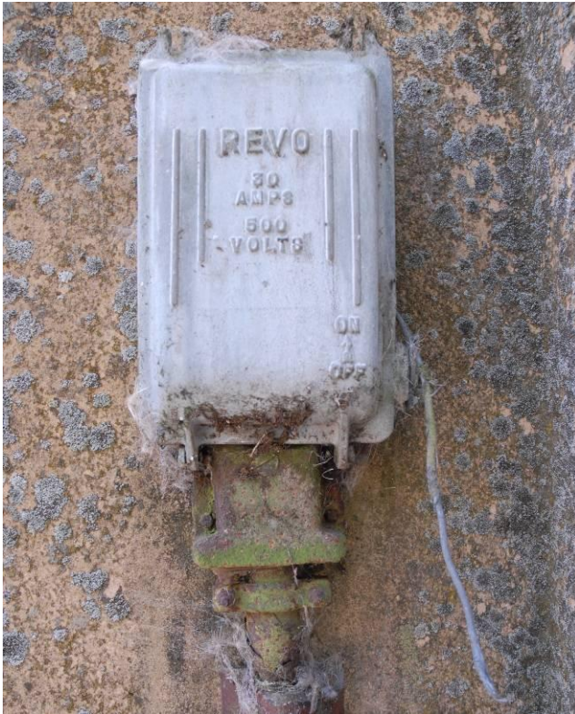
Electric junction box on Hut 141
