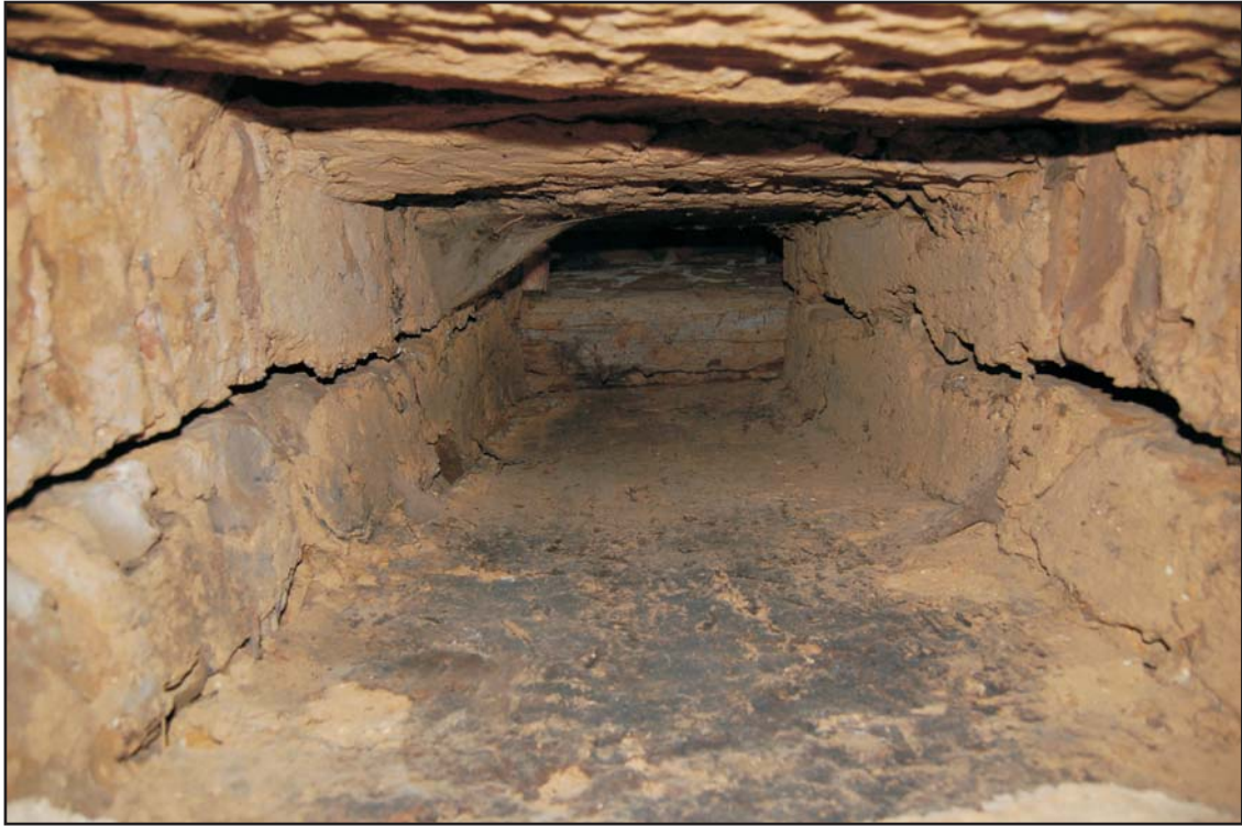
The detached stable fireplace flue, looking up, showing sooting Plate 13
