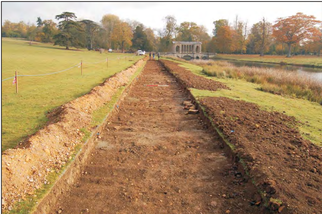
The Octagon Lake path trench, looking east towards the Palladian Bridge from the Chinese Bridge (November 2011)
