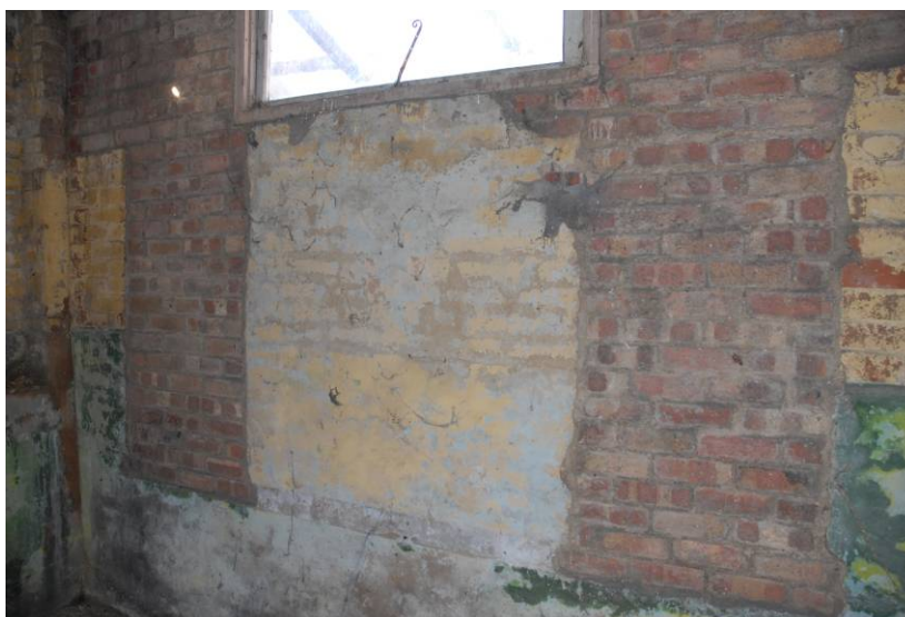
The Cottage, blocked windows at rear of utility room (from west side) Fig 15
