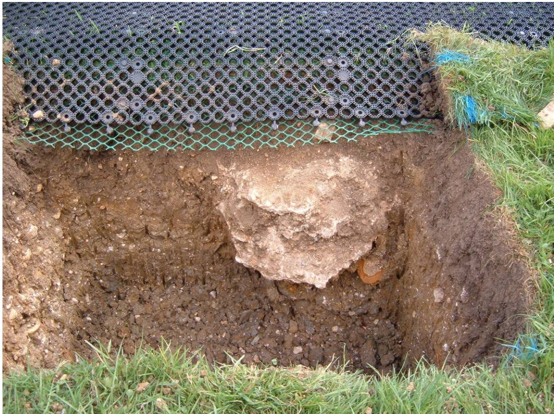
Area 2, north-westernmost foundation, including the concrete base of an earlier piece of equipment Fig 8
