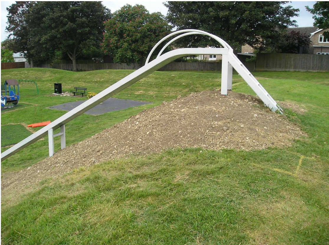
The same erosion covered with excess natural spoil and imported topsoil Fig 12
