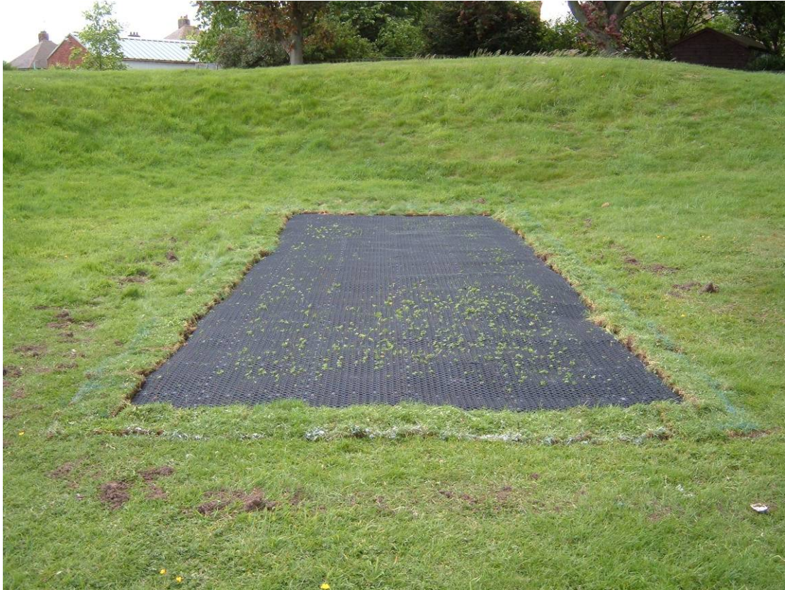
Area 2, an example of the safety matting after the edges have been buried Fig 7
