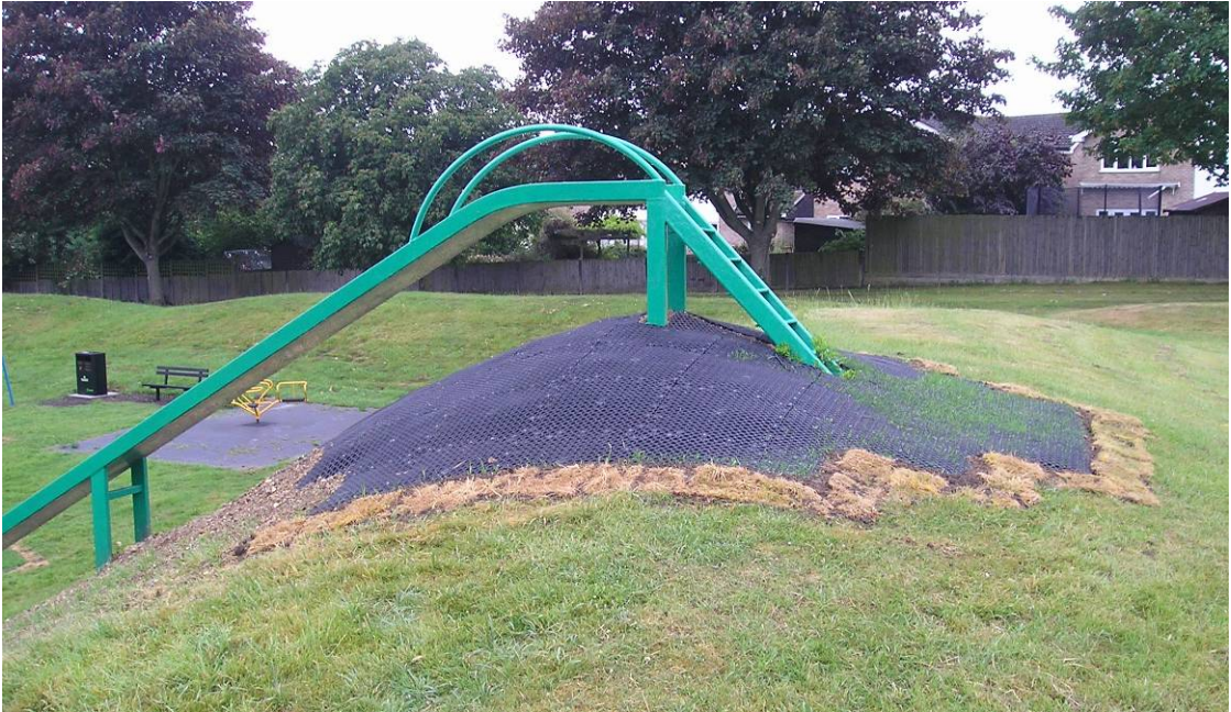
The erosion mitigation works completed by the installation of safety matting Fig 13
