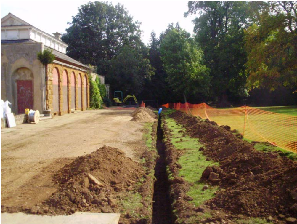
General view of the excavations to the south of the walled garden, looking north-east Fig 8
