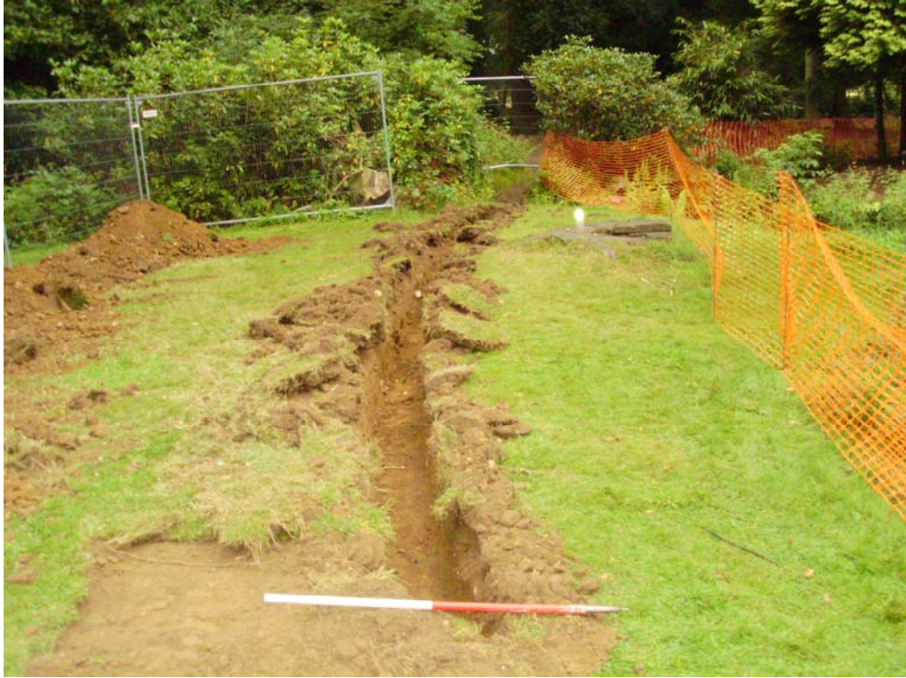
General view of the excavations to the south of the pump pit, looking south Fig 7
