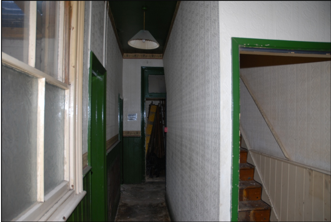
The ground floor corridor with access to the first floor, toilets and passageway Fig 9
