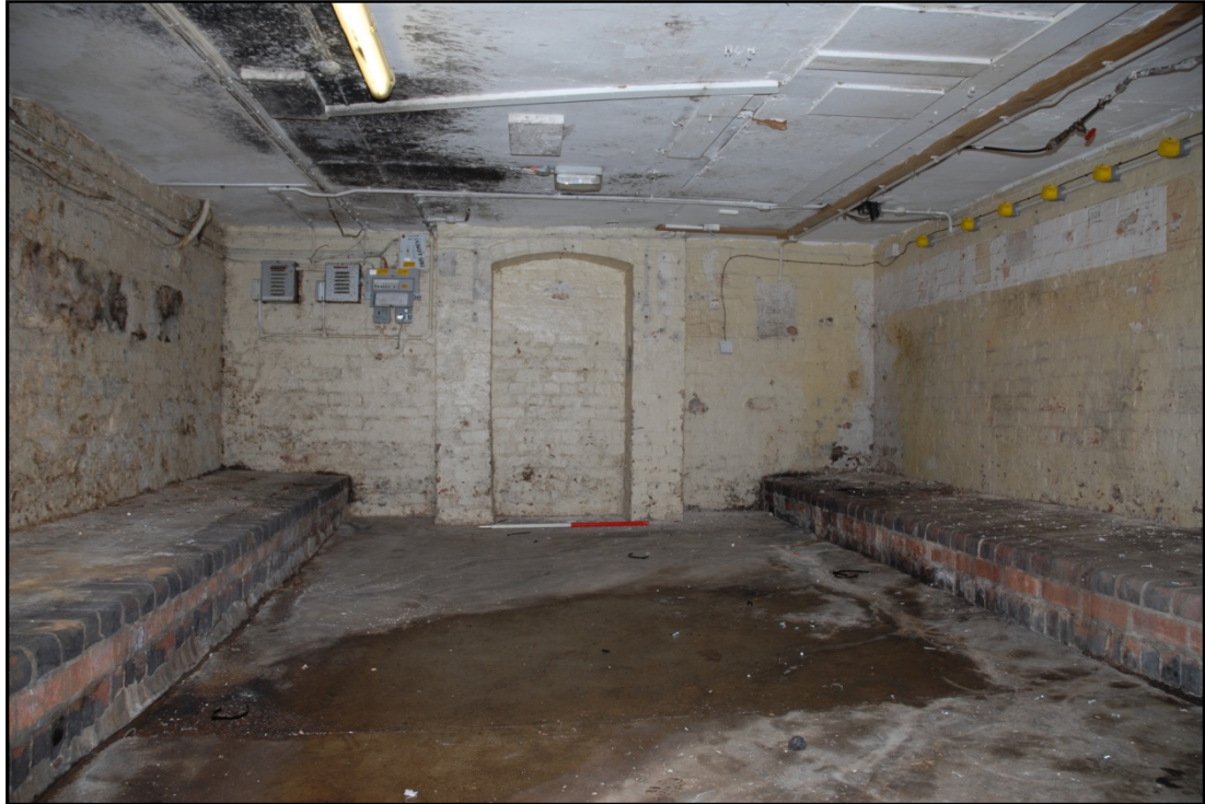
The cellar showing arched recess on the rear wall, supporting chimney Fig 11
