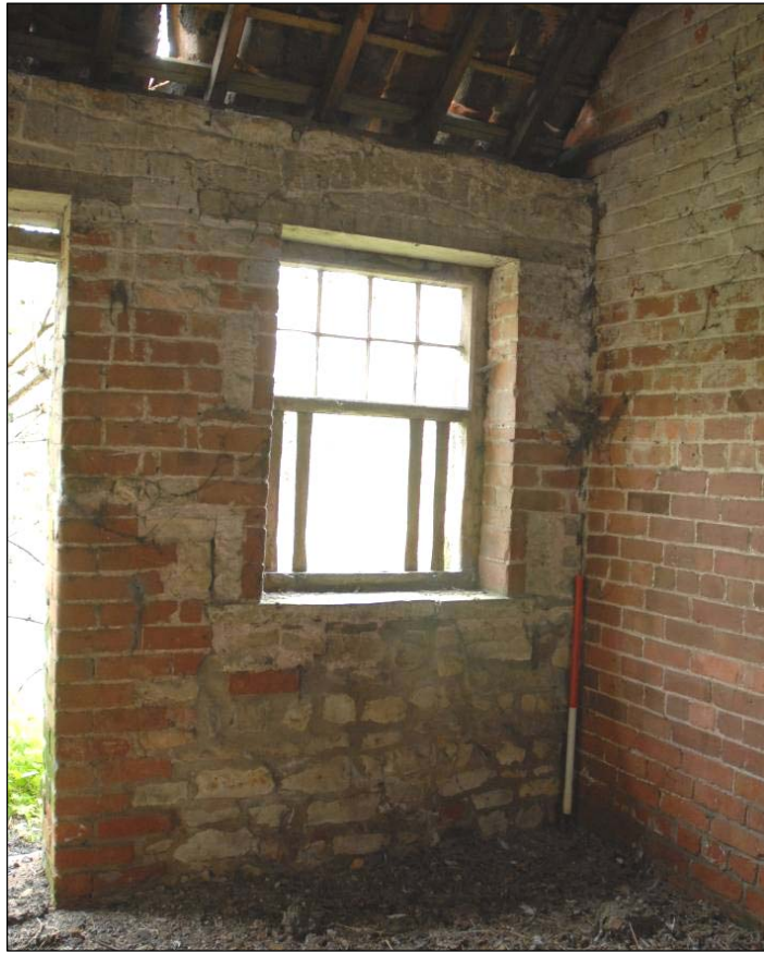
Loose box window, Unit 4
