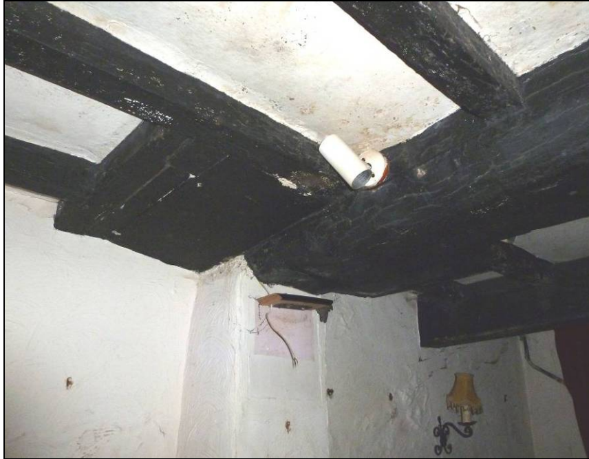
Basement showing exposed beam and joists, with fake beam to the right of the principal beam Fig 15
