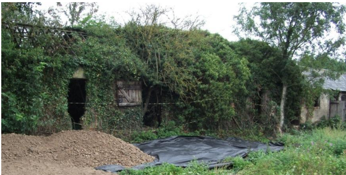
The barns along the north side of the farmyard, looking north Fig 21
