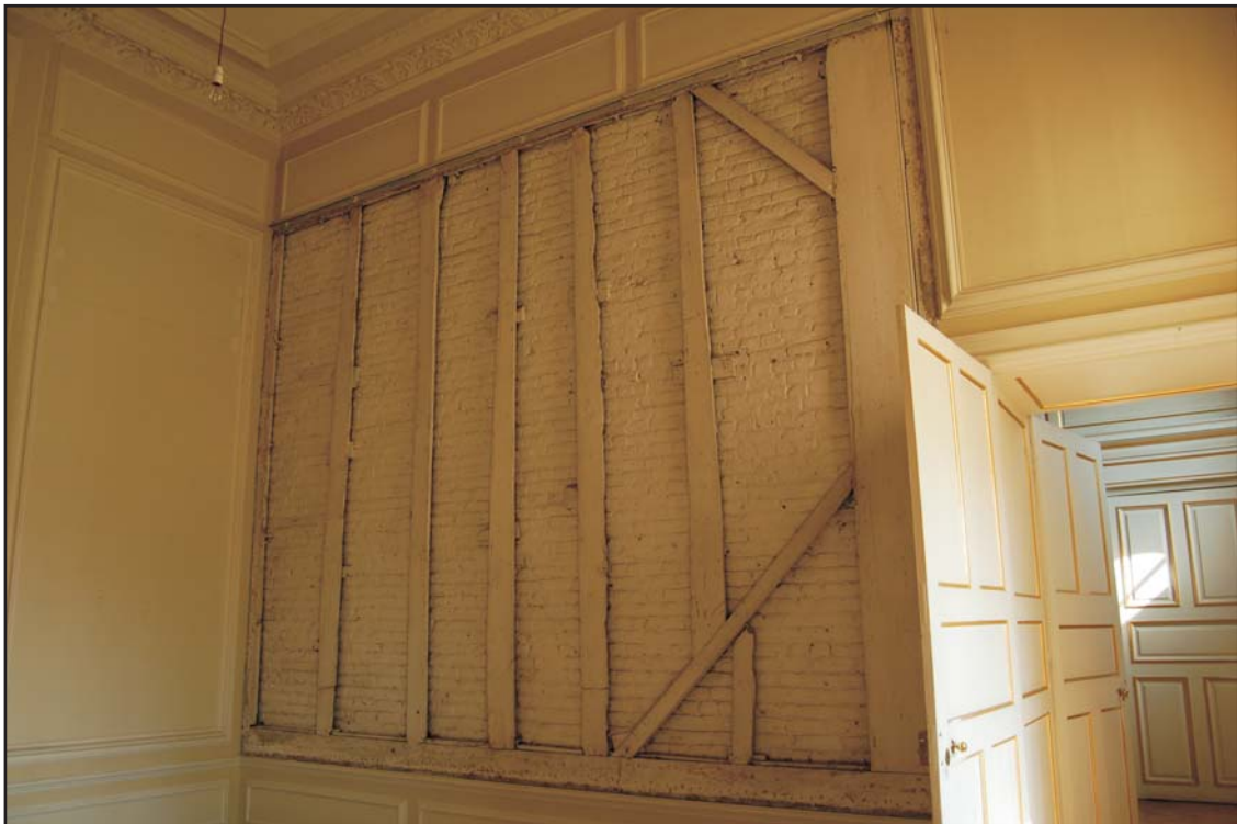
North wall of the first floor Bedroom One showing the location of the former tapestry, looking north
