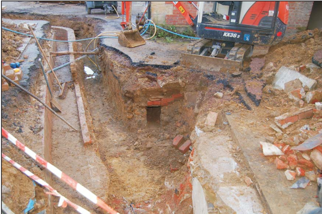
Stone culvert on the north side of the Wren Wing, looking north
