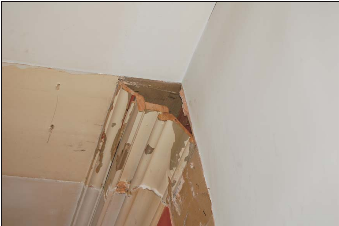
Detail of the timber box-cornice on the south side of the southern room of the kitchen, looking west
