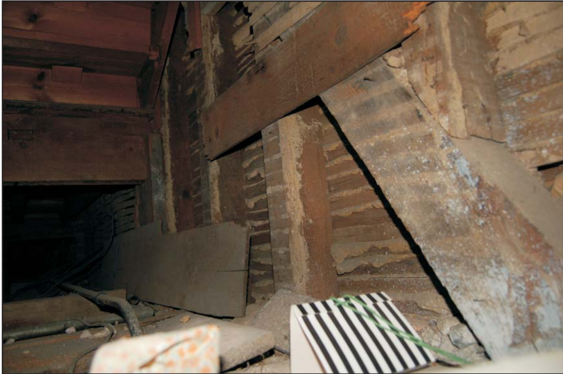
Void beneath raised floor of the corridor to the second bathroom showing back of plaster wall located to the north, looking west
