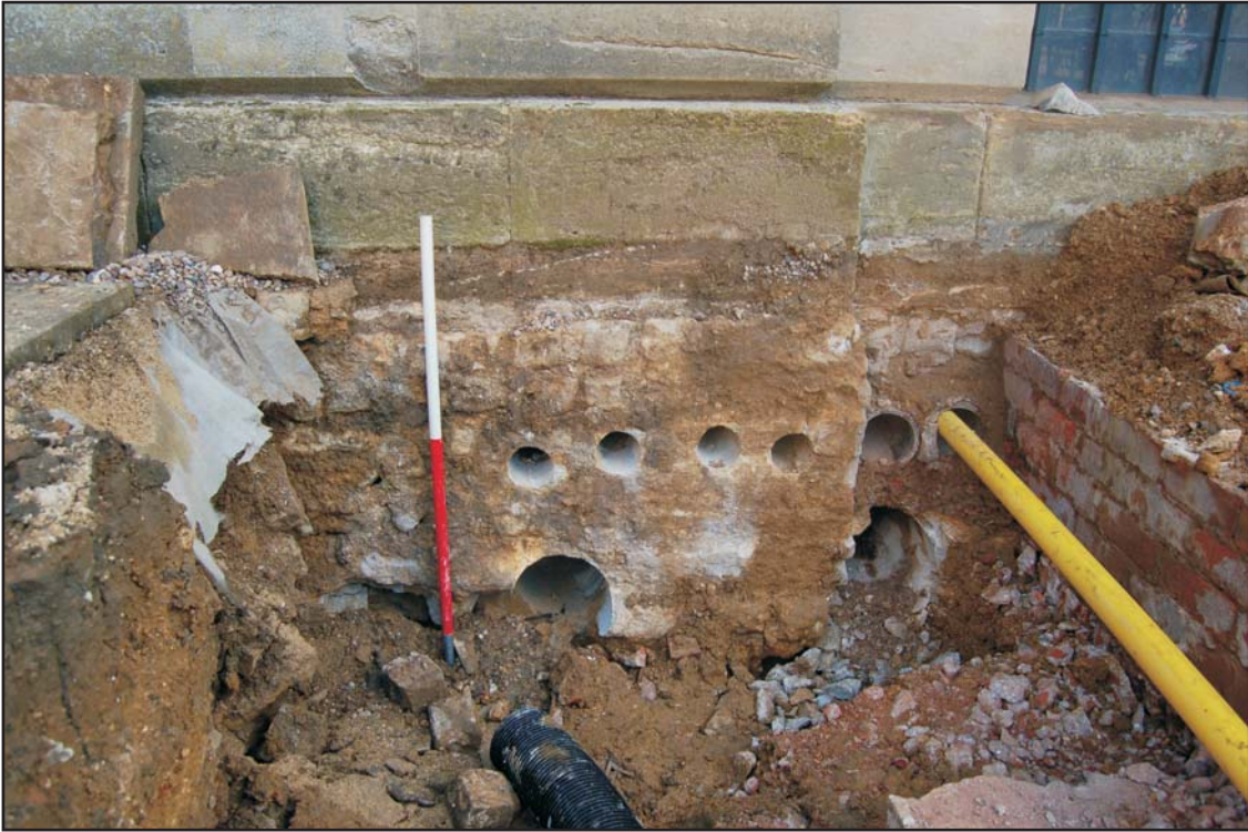
West side of the main house foundation showing drilled holes for new services, looking east
