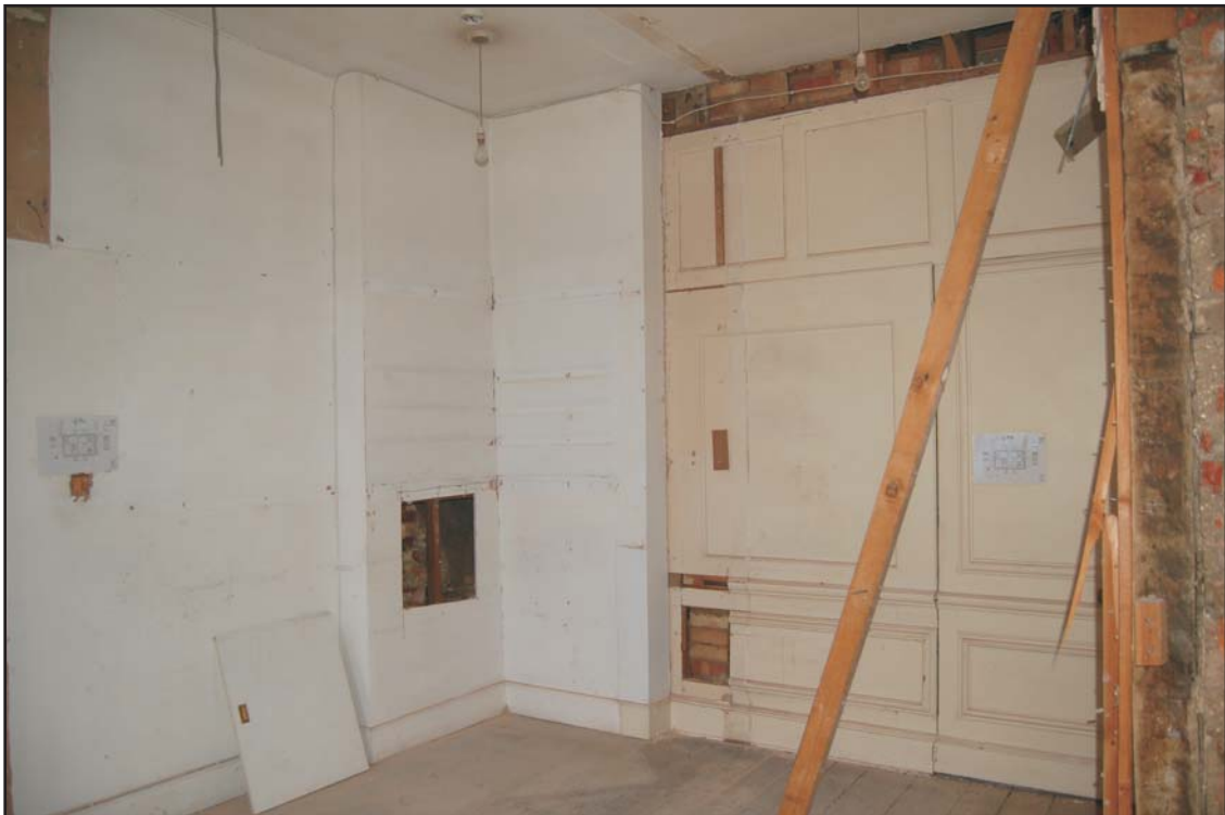
West wall of the southern room of the kitchen showing panelling and jib door, looking south-west
