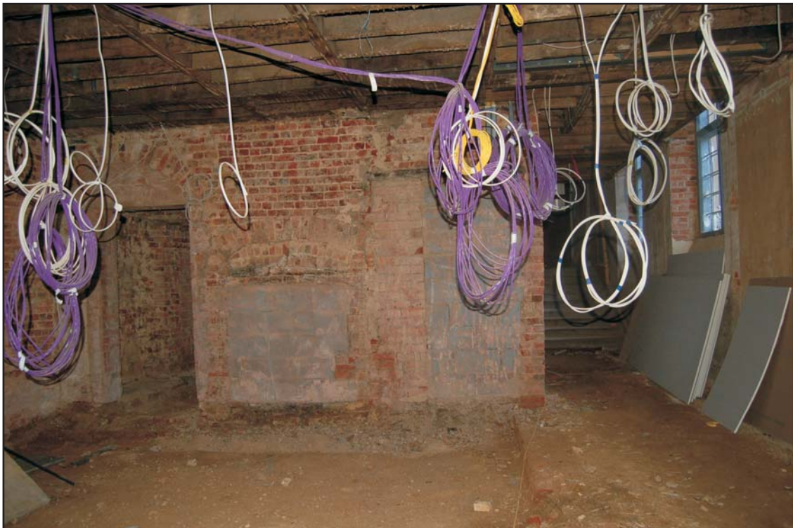
Blocked fireplace (left) and doorway (right) in the east wall of the room to the east of the central doorway in the Wren Wing, looking east
