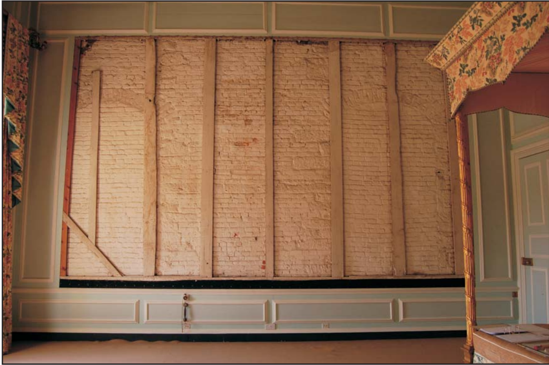
South wall of the Master Bedroom on the first floor showing the blocked arch windows and frame for former tapestry, looking south
