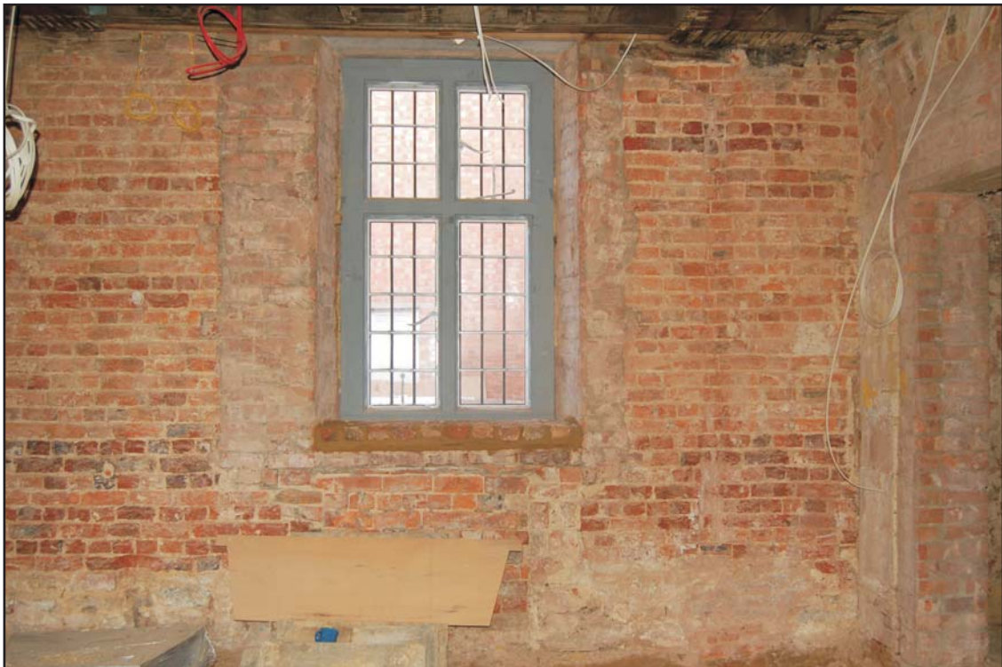
Narrowed window in the north wall of the room to the east of the central doorway of the Wren Wing, looking north
