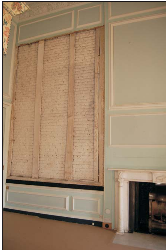
North wall of the Master Bedroom on the first floor showing the location of the former tapestry to the west of the fireplace, looking north
