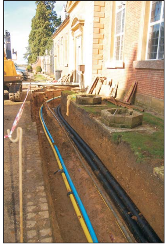
Service trench in the main forecourt of the house, looking west along the south side of the Wren Wing Plate 22
