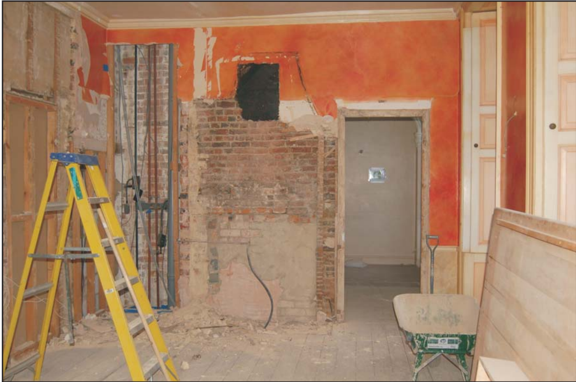
West wall of the northern room of the kitchen showing the blocked fireplace, looking west
