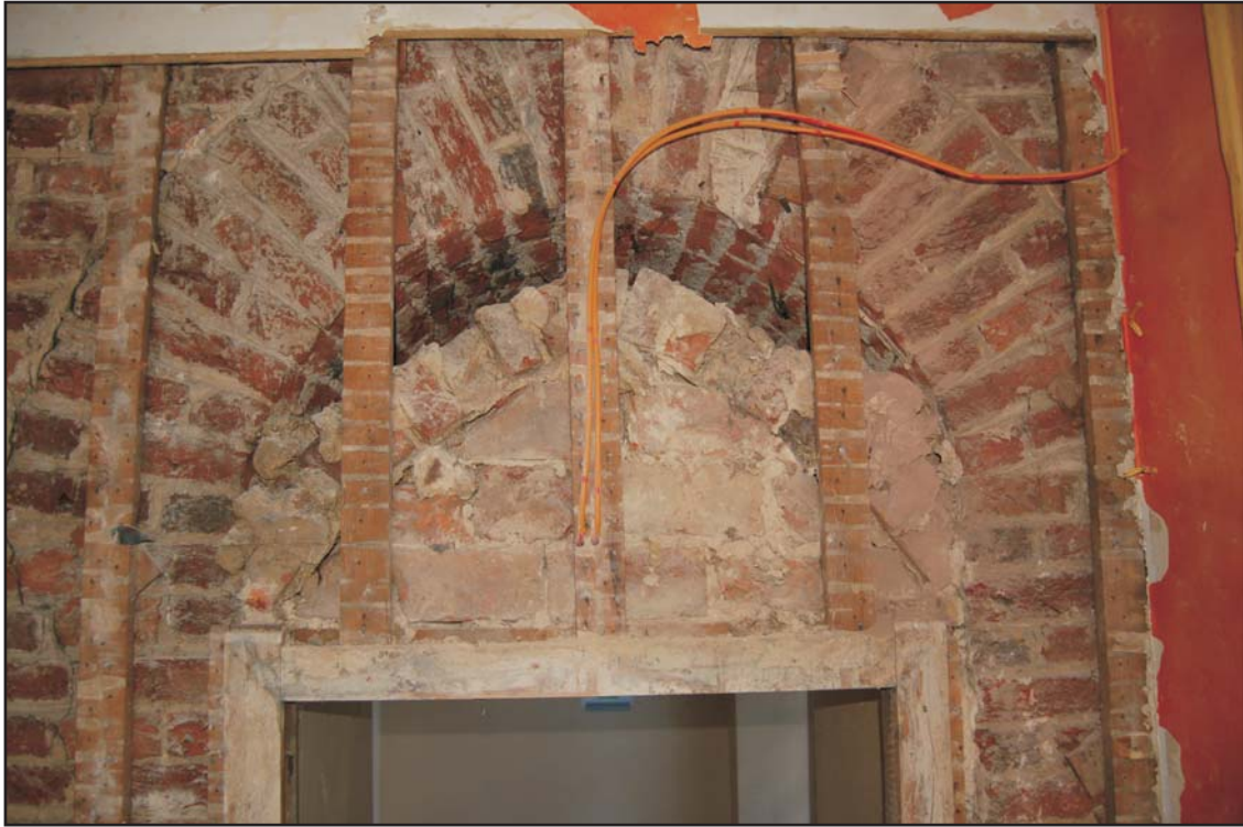
Pointed arch of the vaulted ceiling below the semi-circular structural arch in the west wall of the kitchen, looking west
