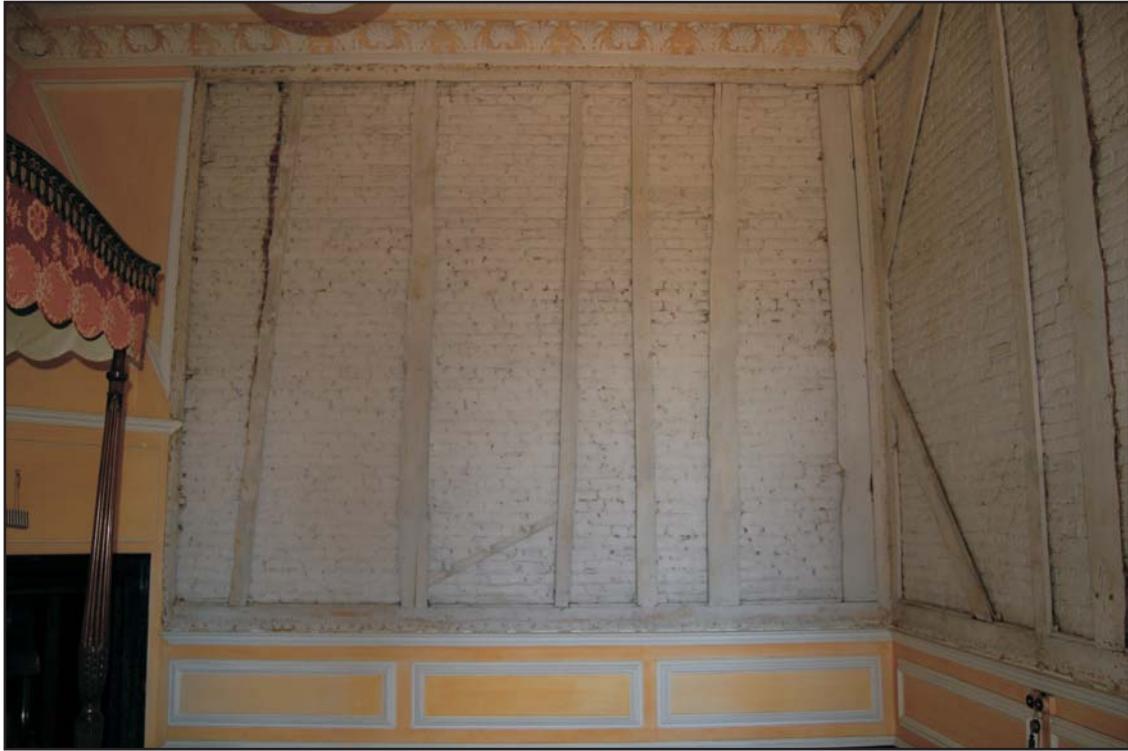
East wall of Master Bedroom Three showing the location of the former tapestry, looking east
