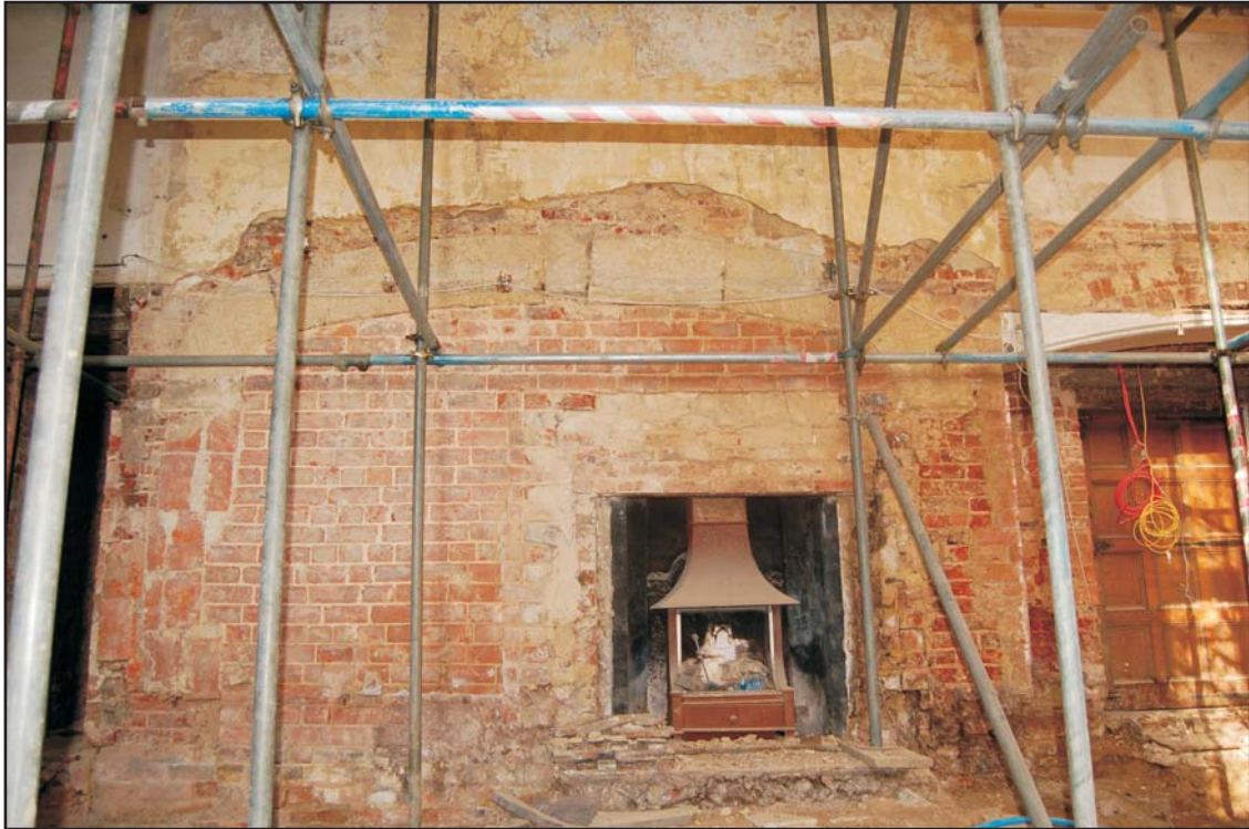
Large fireplace opening with stone voussoirs, subsequently infilled and reduced in the west wall of the service room at the east end of the Wren Wing, looking west
