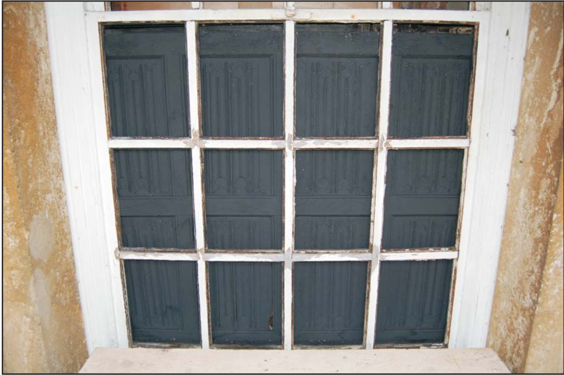
Black painted oak panelling behind glazing bars in the blind window in the north elevation of the main house, looking south
