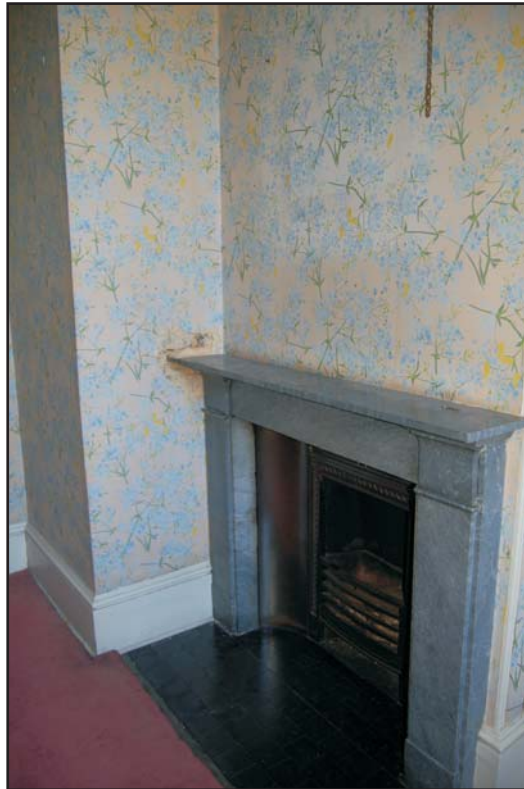
Shaft of dumb waiter built over mantel shelf of fireplace in the west wall of Bedroom Four, looking west
