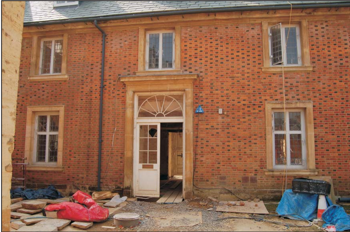
Exterior of the north wall of the Wren Wing showing evidence of the re-facing with new brick and stone surrounds to windows and doorway, looking south
