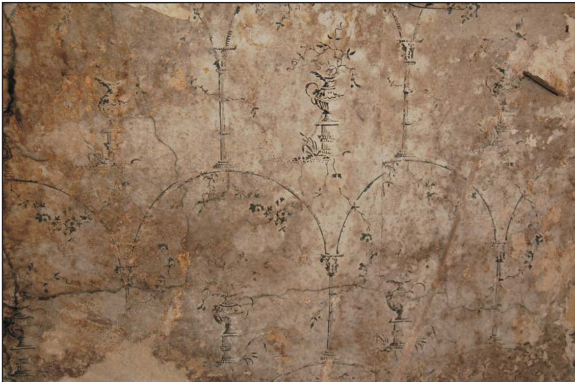
"Pillar and arch" pattern wallpaper of c1775-1780 lining archway formerly overlooking the full height hall
