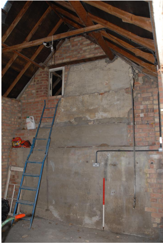
The rear of the chimney structure in the modern garage extension Fig 6
