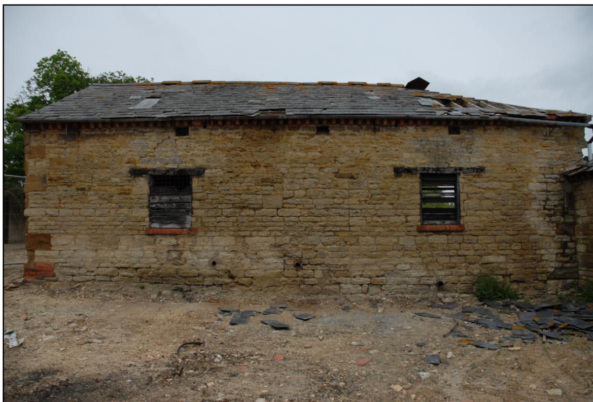
The blocked door on the southern elevation of building B3, looking north-west Fig 25
