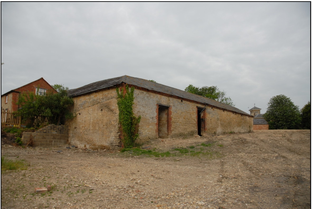
The southern elevation of building B1, with the scar of a former building visible to the left, looking north-west Fig 13
