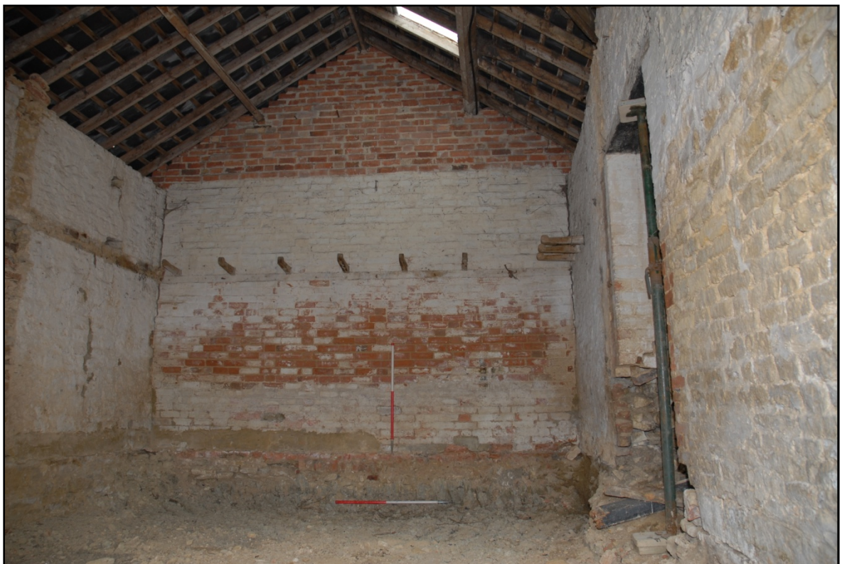
Room G2 showing the scars from a removed partition and former hay loft, looking south-west Fig 15
