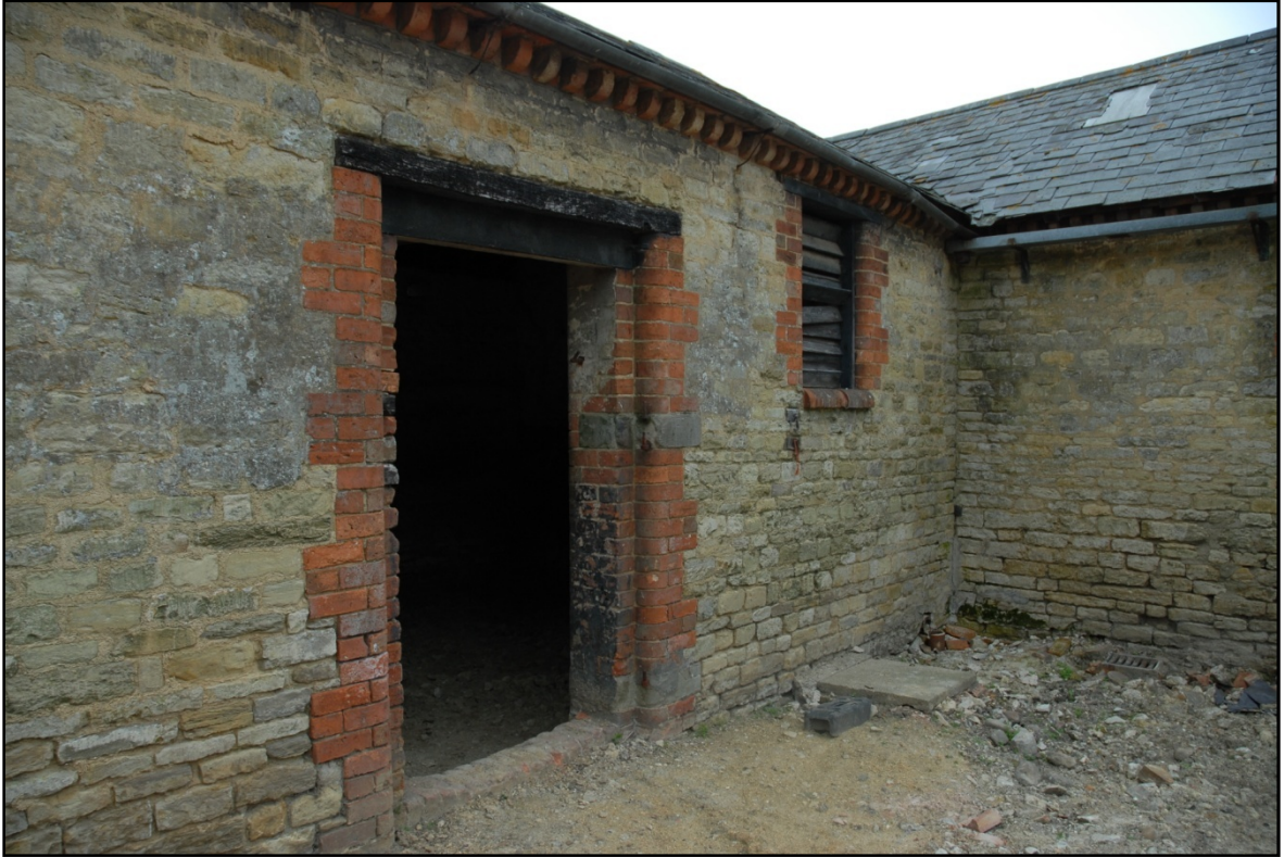
Detail showing the construction of the doors and windows, also showing the inverted bullnose dentils Fig 22
