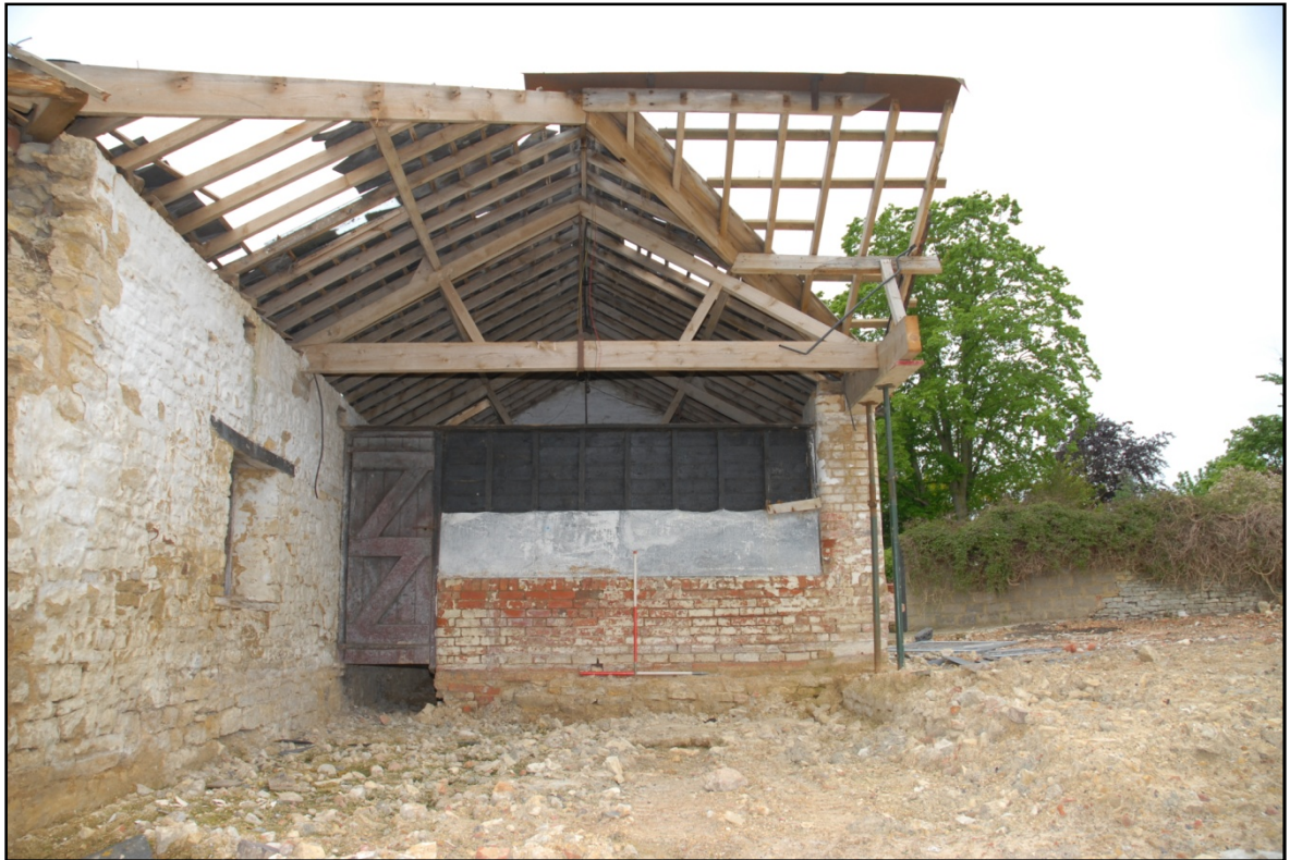
Room G6 showing the inserted half wall and timber partition, looking south-west Fig 20
