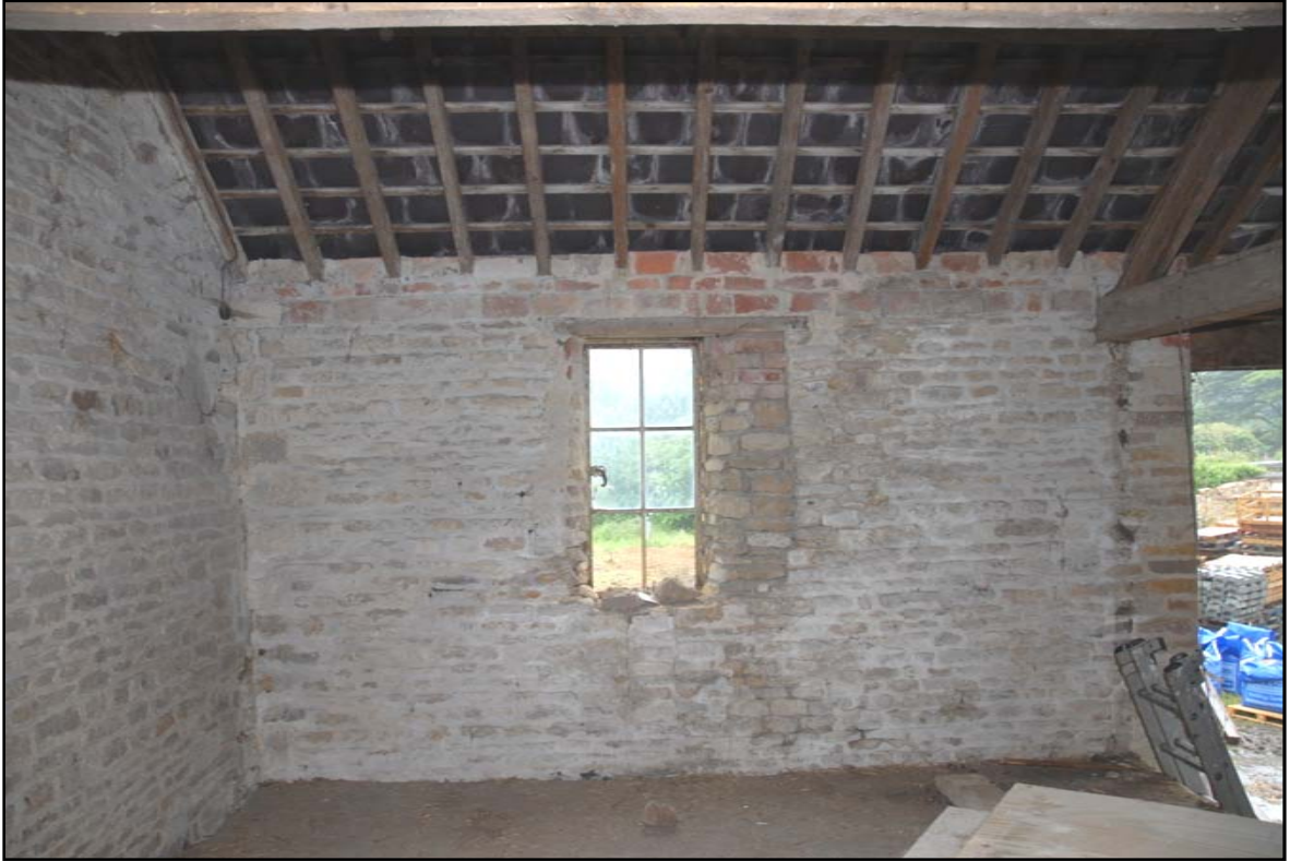
Room F1 showing the altered window with scar of former boarding visible to the right, looking south Fig 24
