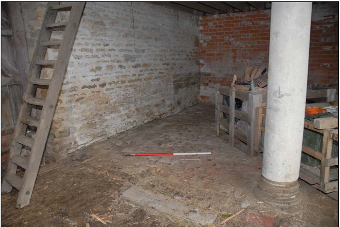
The threshing floor and the floor of Room G1 with the column to the right Fig 13
