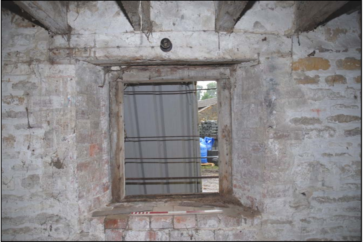
The window in G2 with floor joists resting on the lintel Fig 18
