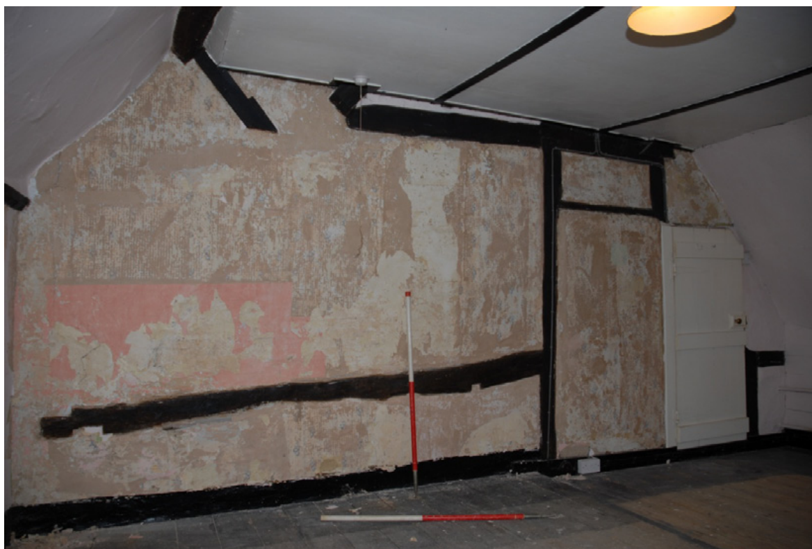
The west wall of Bedroom 1 showing the timber frame and defunct lap joints in the horizontal timber Fig 53
