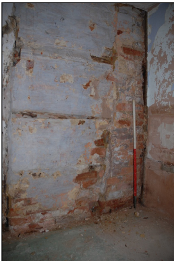
The east partition wall abutting the south wall in the bathroom showing timber bond Fig 43
