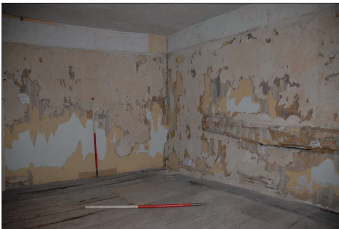
The north-east corner of Bedroom 2 showing the trapdoor and timber beam in the east wall Fig 56
