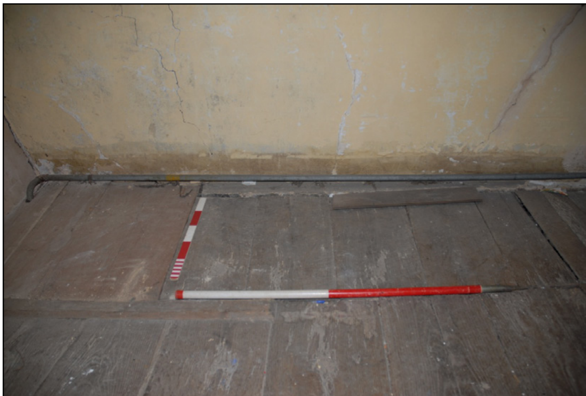
The raised floor boards at the north end of Bedroom 4, with trapdoor to the left Fig 64
