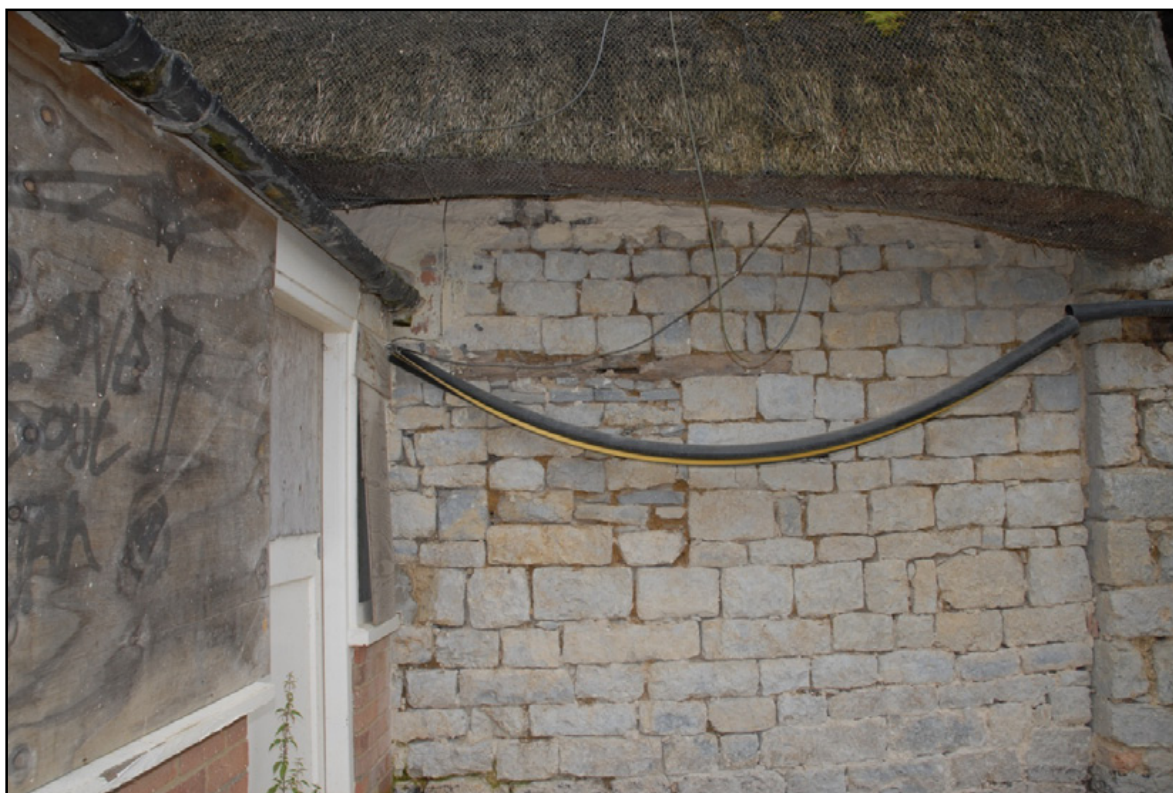
The blocked window Fig 13
