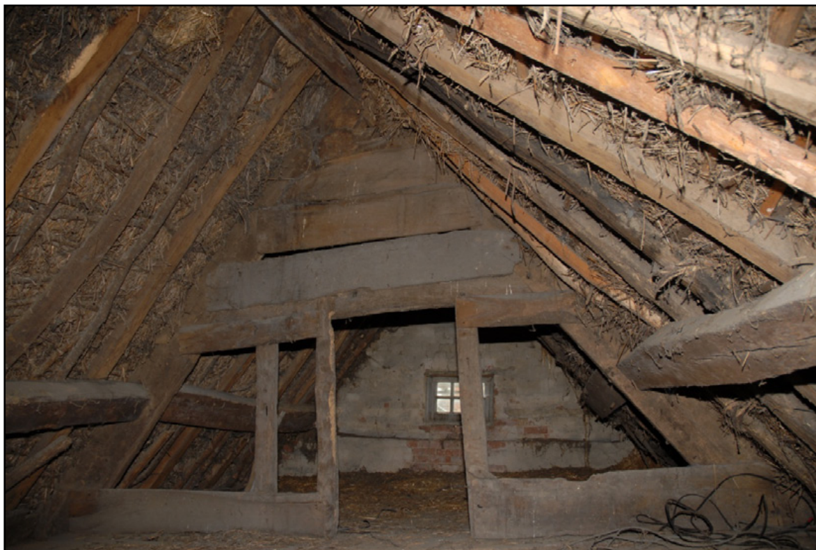
The modified queen post truss, looking west toward the west gable Fig 65
