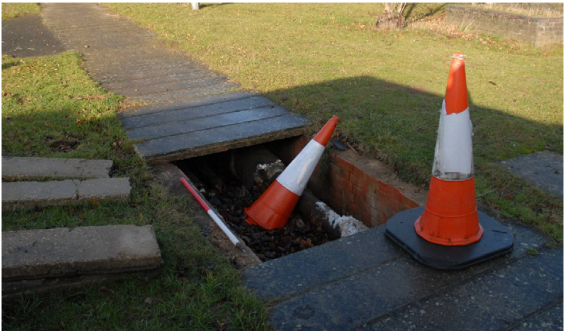
Ducting for pipes Fig 8
