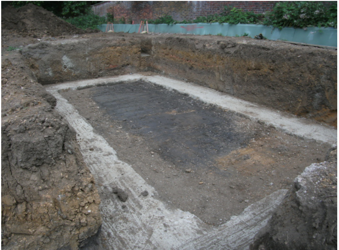
The foundations in the area of the new swimming pool, looking north-east Fig 6
