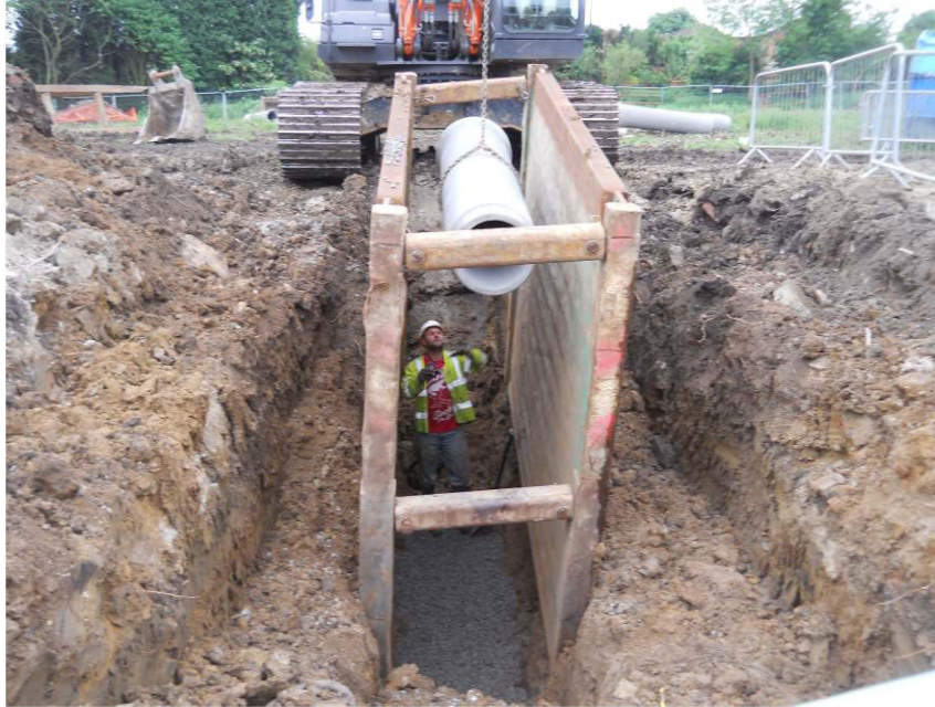
Metal shuttering in the deepest part of the sewer trench, looking south Fig 4
