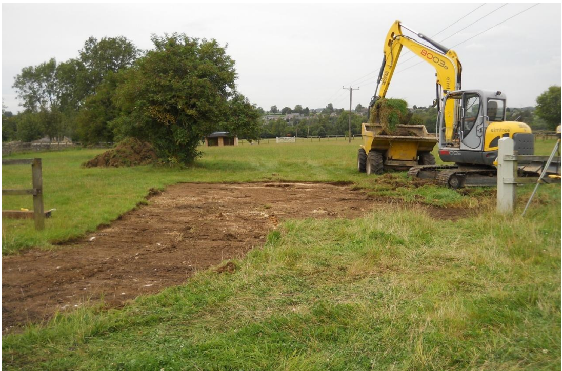
Topsoil removed from new access road going into ménage area, looking north Fig 4
