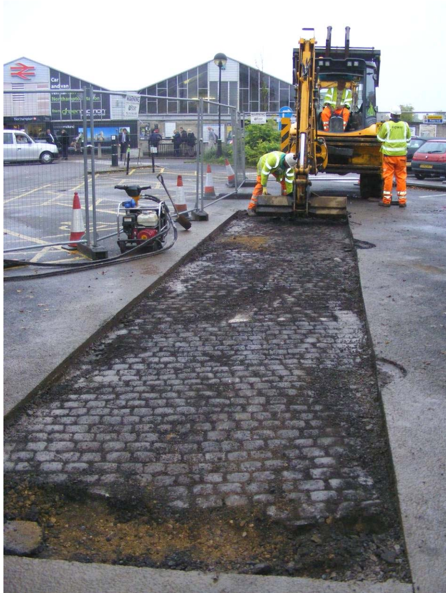
The granite setts of the old station yard, covered over in 1964 Fig 16
