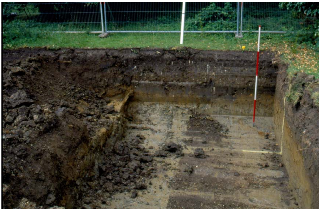
The area of the new swimming pool after excavation, looking south Fig 8
