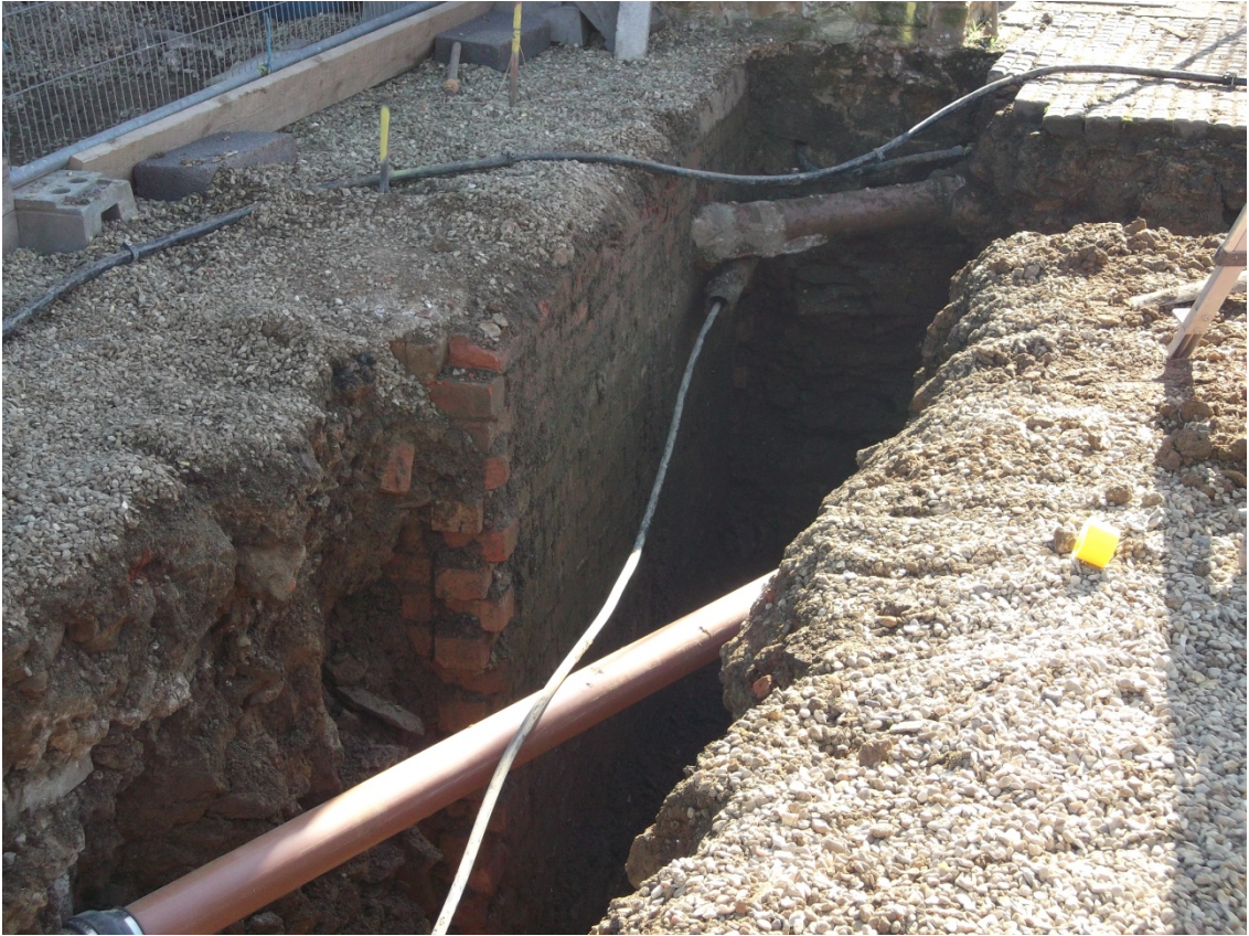
The water-tank and modern services Fig 6
