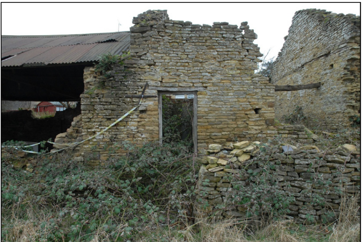
The north elevation of Room 2, showing the doorway and iron tie, looking south-east Fig 20
