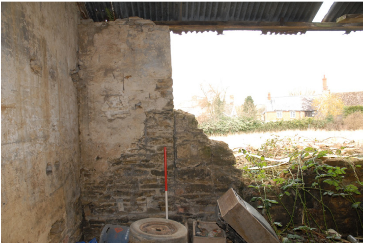
The vertical joint beneath the window opening on the northern wall, looking north-west Fig 14
