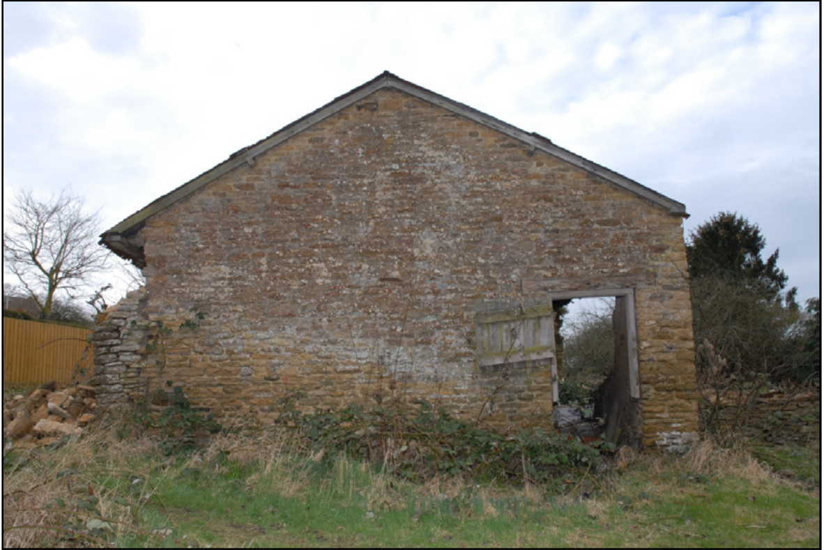
The eastern elevation, showing differential weathering, looking south-west Fig 7
