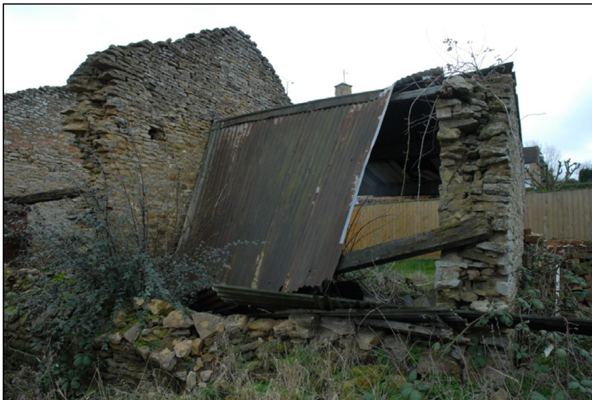
The north elevation of Room 3, showing the collapse of the north wall and roof Fig 22
