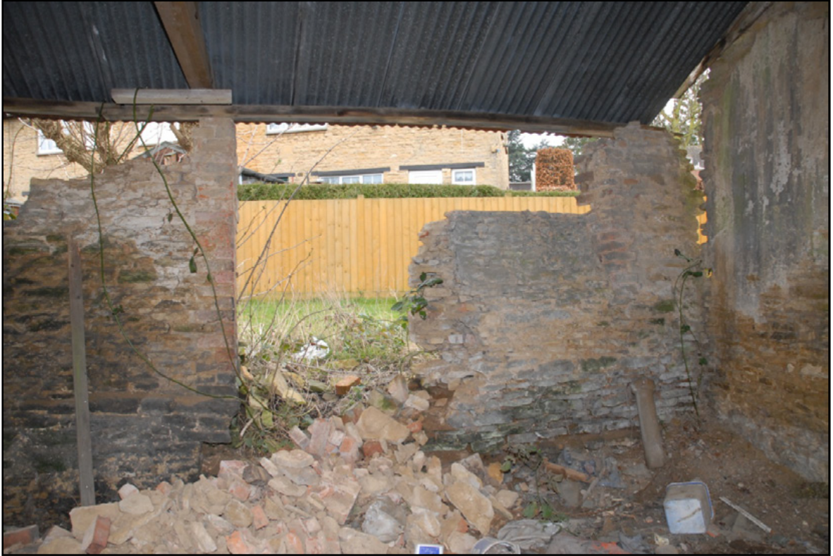
The doorway and window opening on the southern elevation of Room 1, looking south Fig 13
