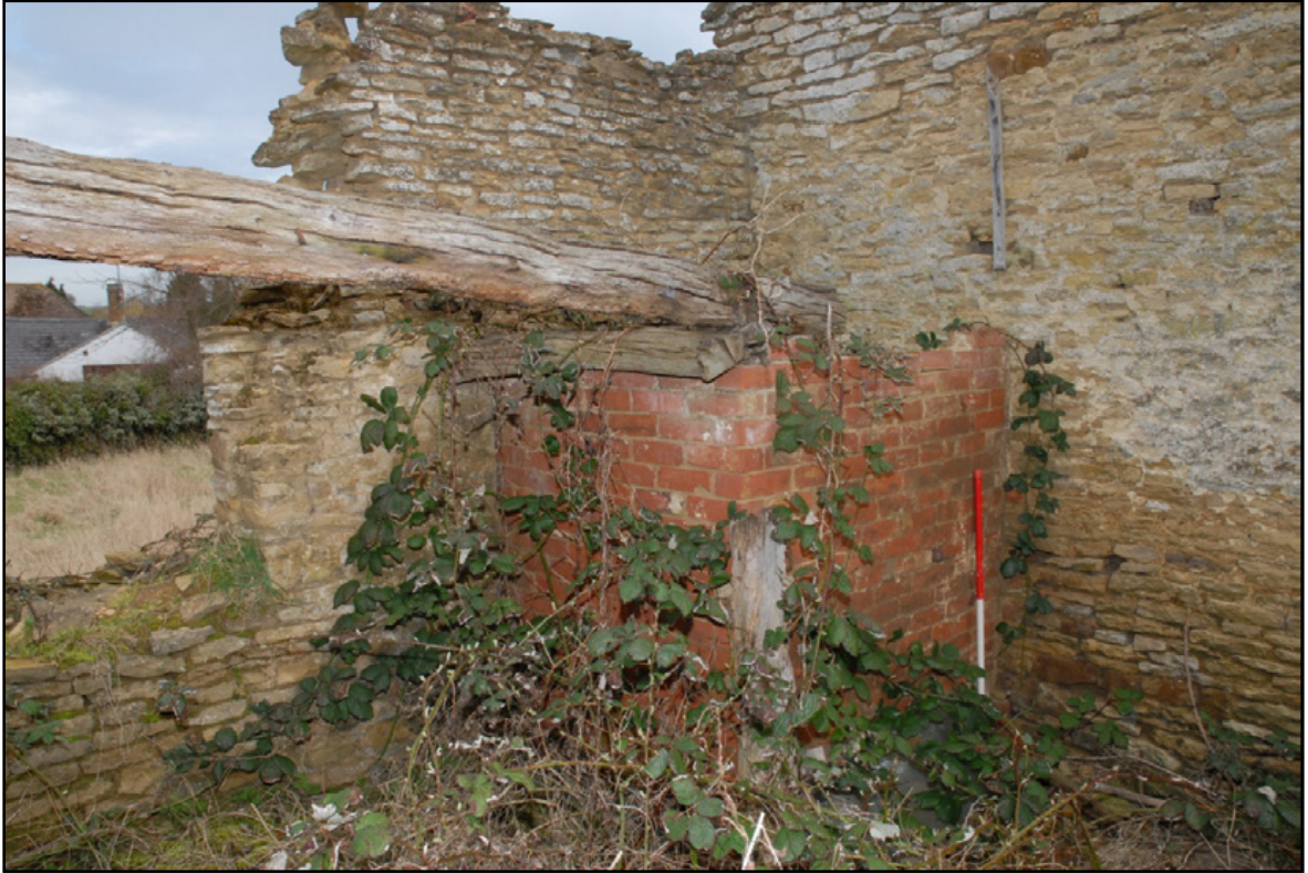
The brick partition with extraneous timber and the tether post obscured by vegetation, looking north Fig 17
