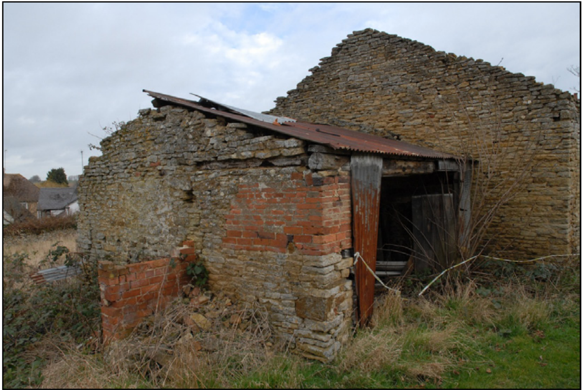
The west elevation of Room 3 with the wall of Room 4 to the left Fig 27
