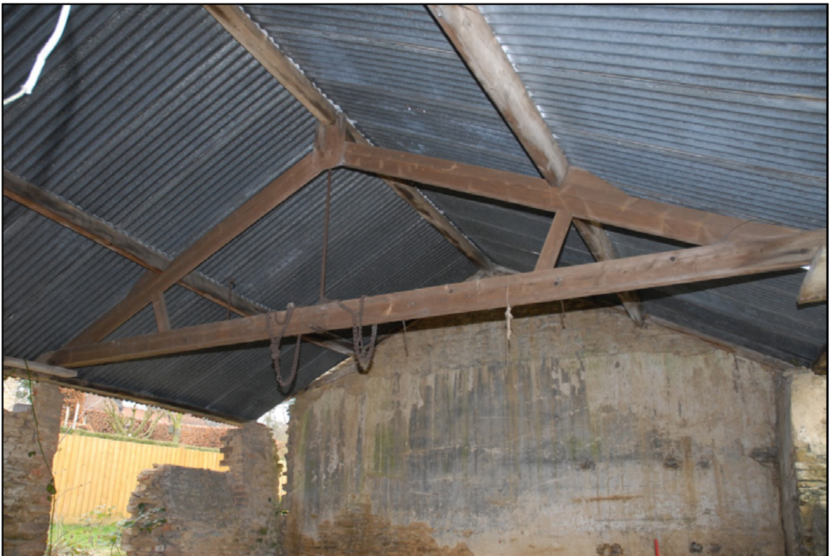
The corrugated iron roof with wooden frame, truss and supporting rod Fig 12
