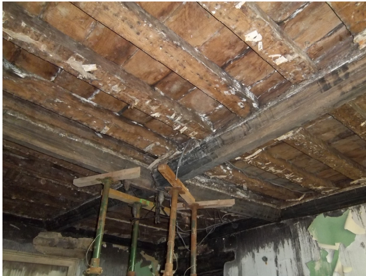
Figure 3a/b/c: Views of the in-situ truss to the north range (top), the ex-situ timbers salvaged from this roof (middle), and the ground floor ceiling beams (bottom)
