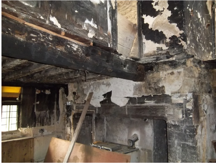
Figure 3g: Views of the kitchen ceiling beam and fireplace bressumer to the ground floor of the south range
