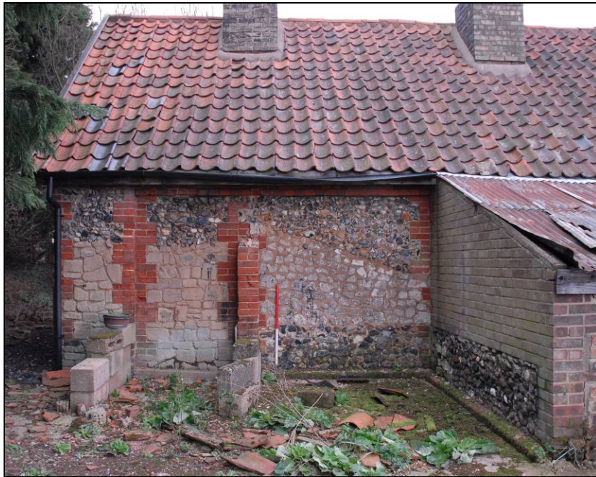
Rear elevation, looking east, showing the panels of limestone and chalk blocks Fig 12
