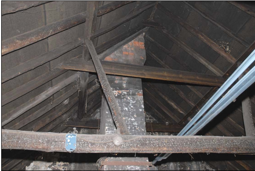
Roof structure, looking north, showing tie-beam, brace supporting the purlin, and the collar-beam between the rafters Fig 19
