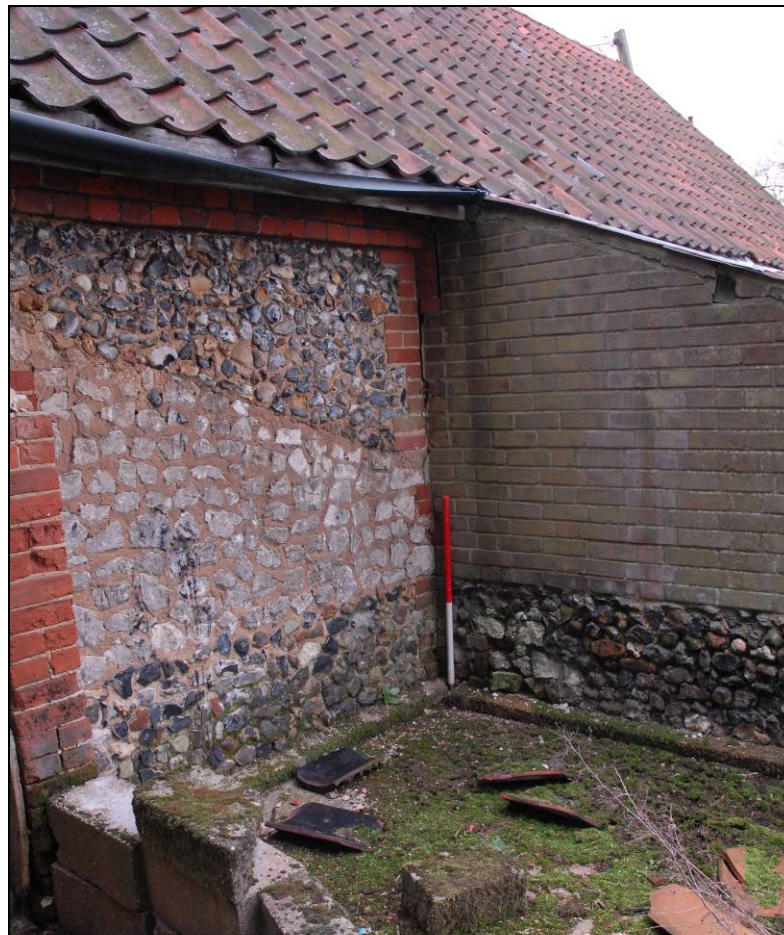
Northern elevation of the lean-to showing the more recent brickwork over the original flint walling, looking south-east
