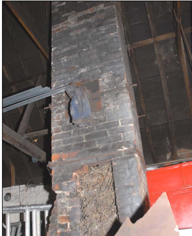
Chimney over the hearth where the smoke hood has been removed Fig 17
