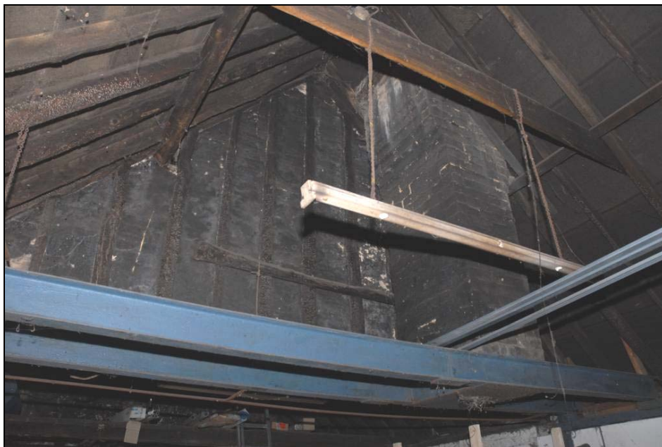
The central chimney looking south-west, supported on RSJ girders, also visible is the lath and plaster partition Fig 15
