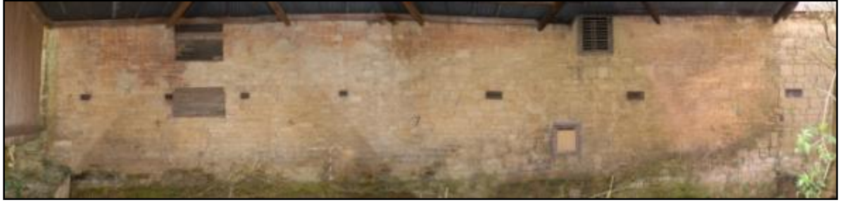
North elevation of the stables and barns as seen from within the Lean-to (Photocomposite) Fig 44
