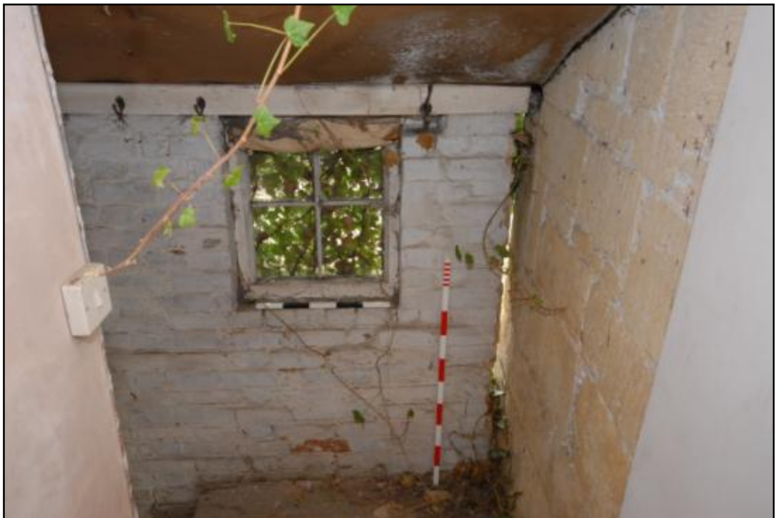
Interior of the stair, showing the join with the main structure Fig 15
