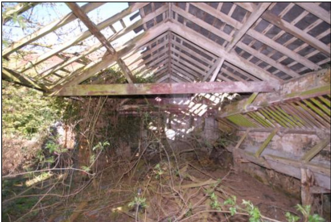
Stable 3, interior, looking north with hay rack and trough to the right Fig 37
