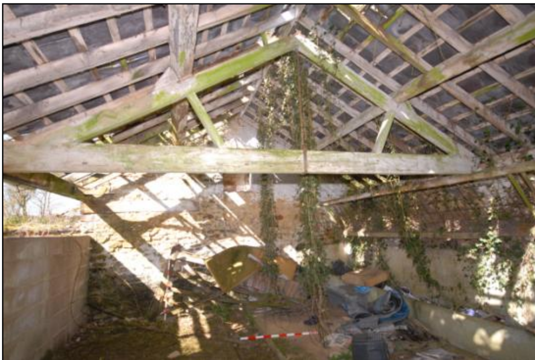
Stable 4, interior, looking west, showing trough and hayrack to the right Fig 40
