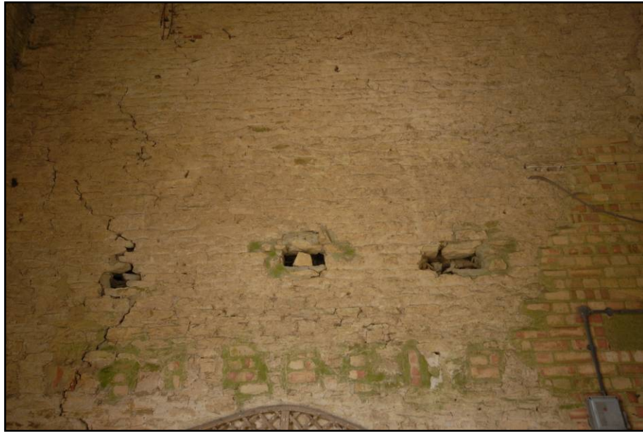
Holes in the wall, looking south-east Fig 32
