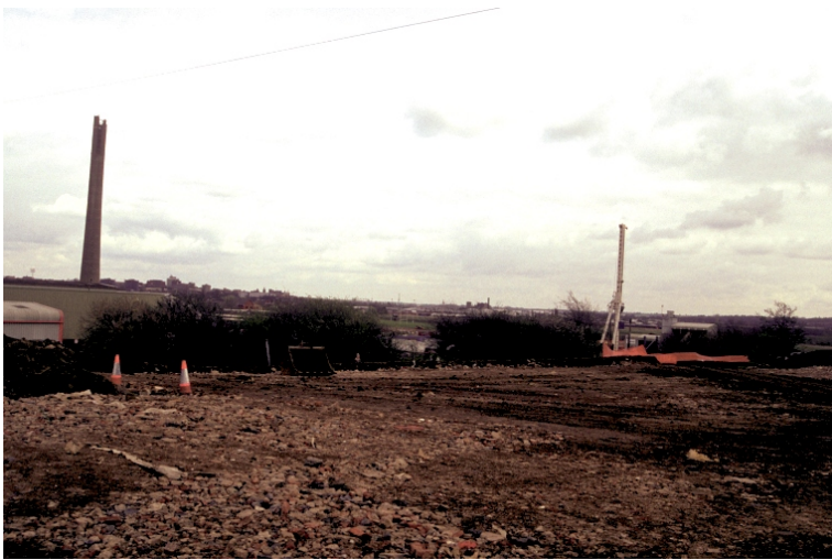
Plate 1: General site shot looking towards Harvey Reeves part of site. Looking east
