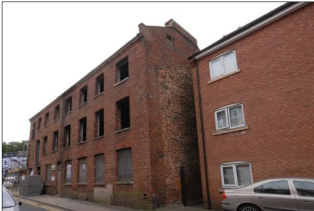
The north and western elevations of Building 2, showing scar of demolished structure Fig 9
