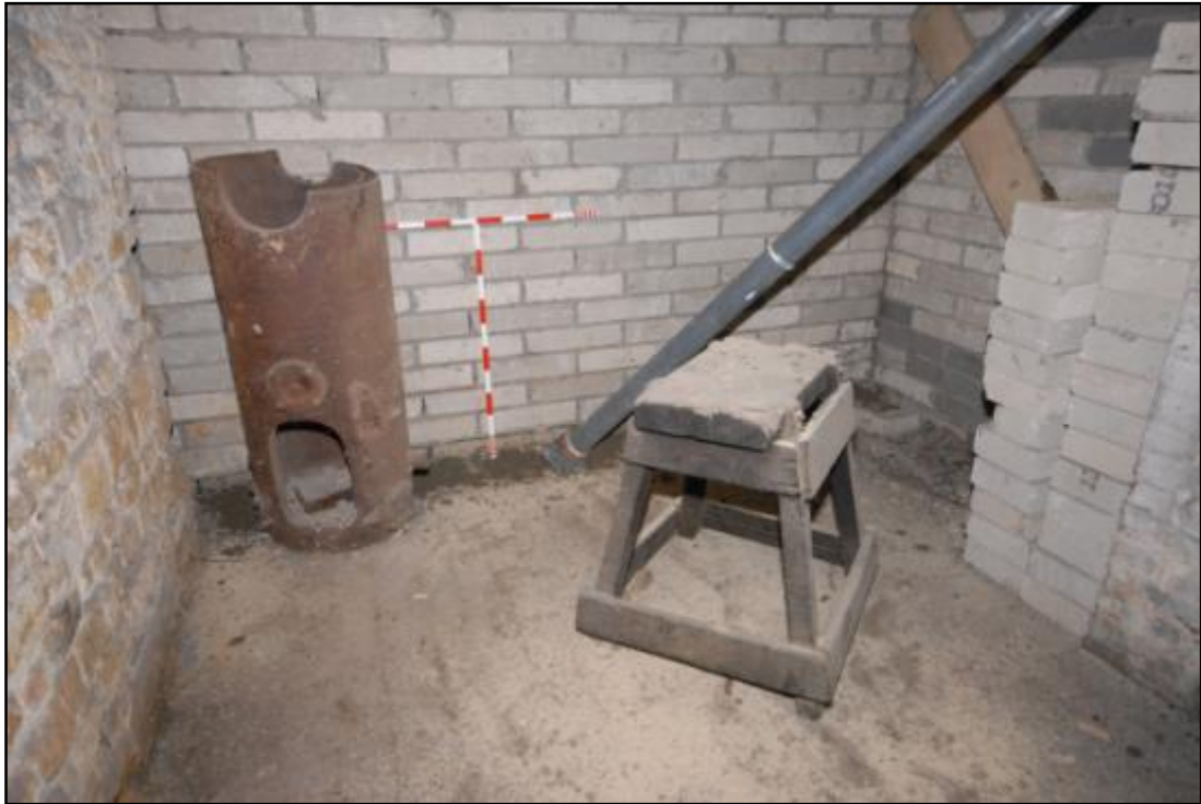
Boiler or heater and work bench in Room B2 Fig 62
