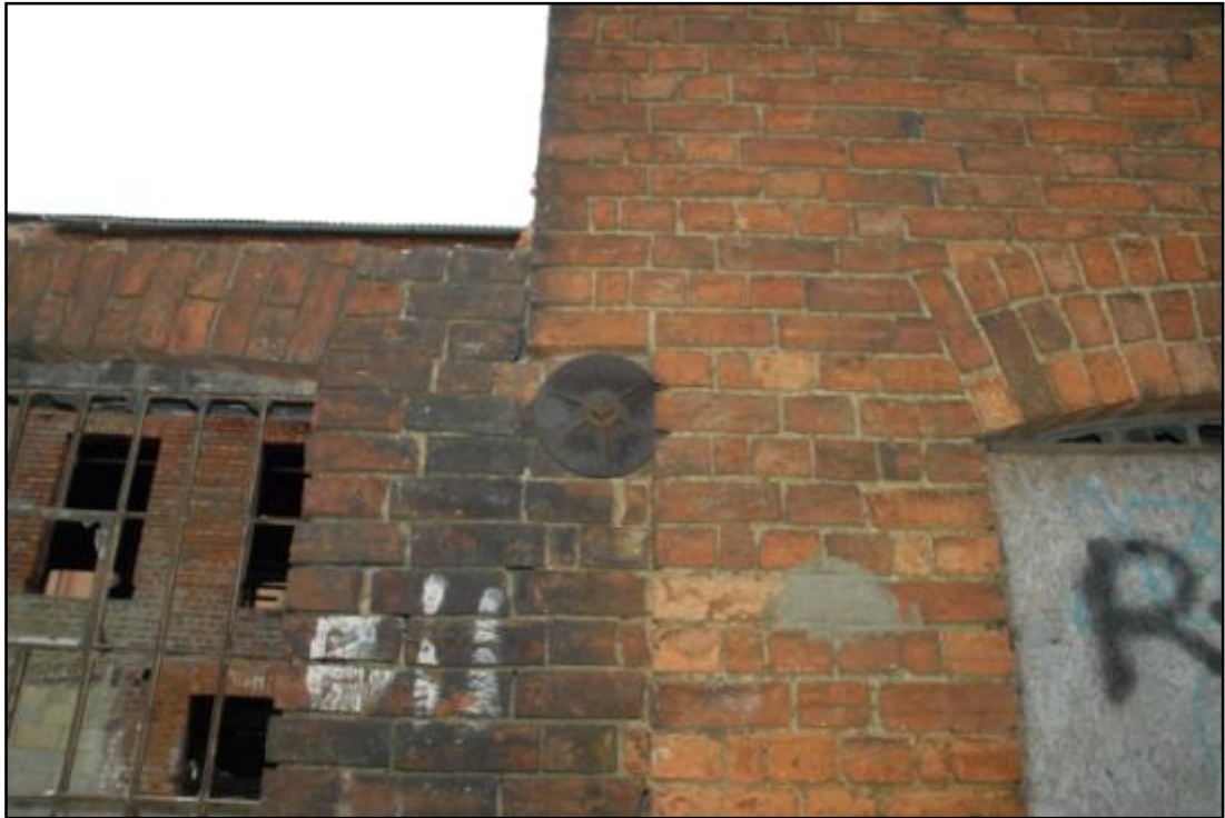
Building 1, south elevation, showing the join between the annex and Building 1 with iron tie plate Fig 24
