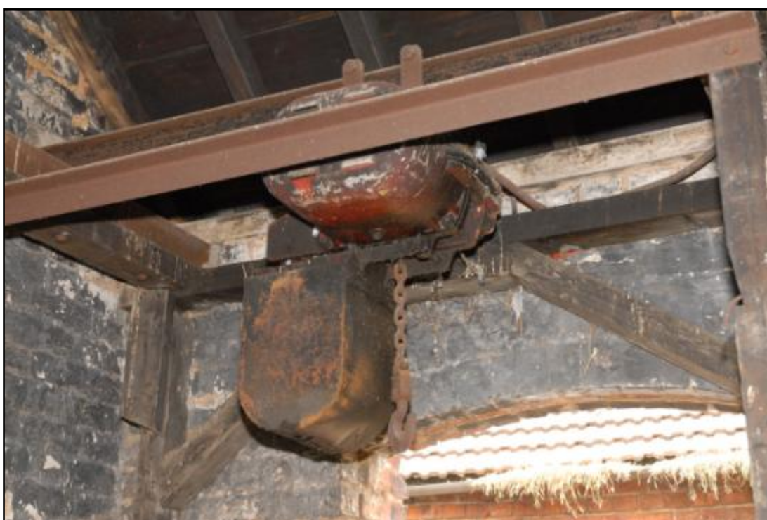
Detail of the lift hoist Fig 41
