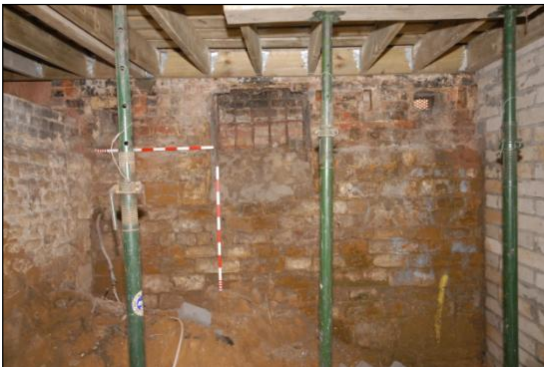
Room B1, blocked light well with vent to the right, looking north Fig 54
