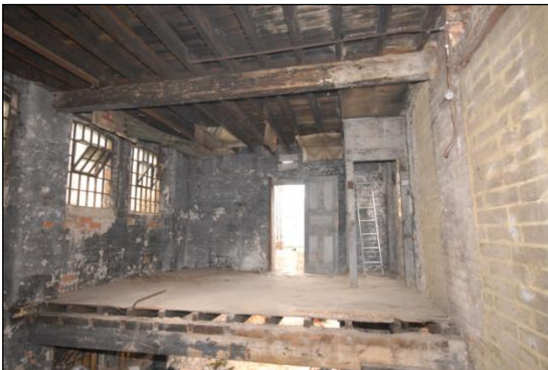
Building 1, first floor, looking west, showing lift shaft and door to former annex Fig 32
