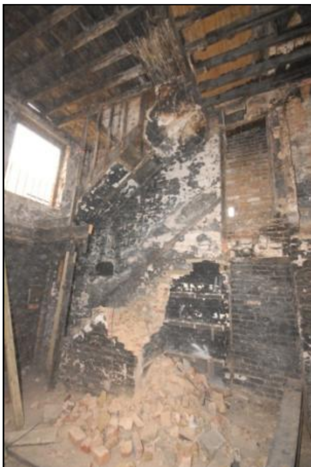
View of the stair from ground to first floor after demolition Fig 46
