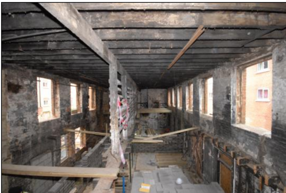
Building 2, first floor, looking west, showing the remains of the central partition and joists Fig 63
