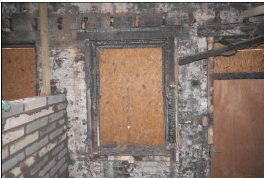
Building 2, ground floor, fire damaged sash window Fig 48
