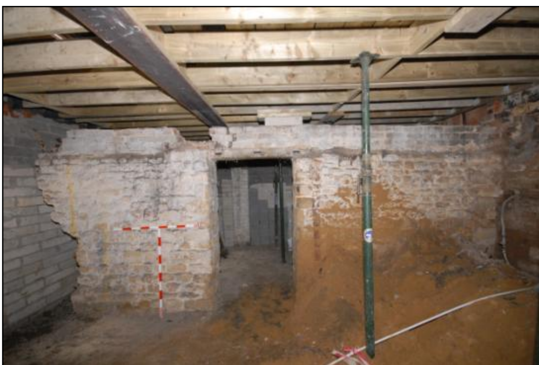
Room B1, the central basement partition wall with door through, looking west Fig 53
