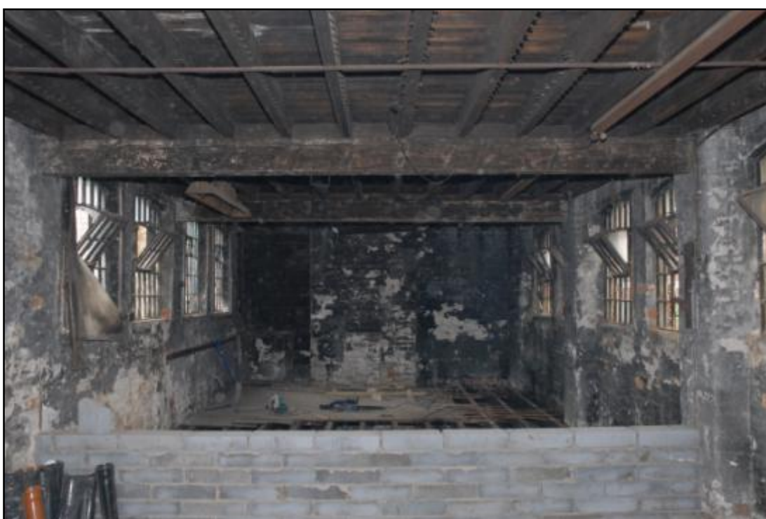
Building 1, first floor, looking east, showing chimney flue with blocked fireplace Fig 33
