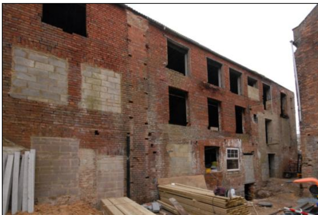
South elevation of Building 2 with staggered beam slots and scar visible, looking north- east Fig 17
