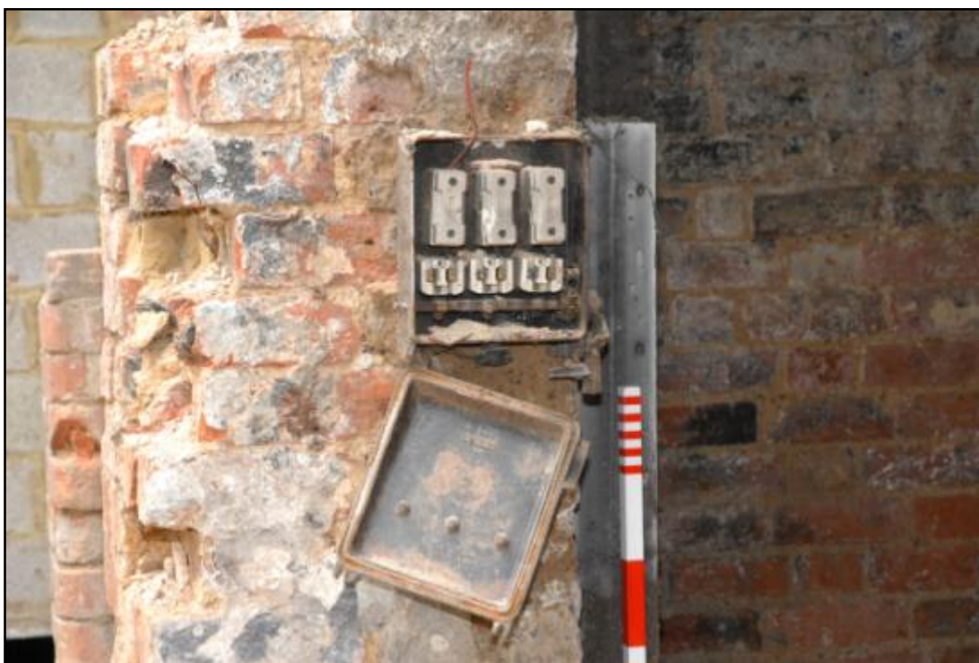
Detail of the electric box Fig 31
