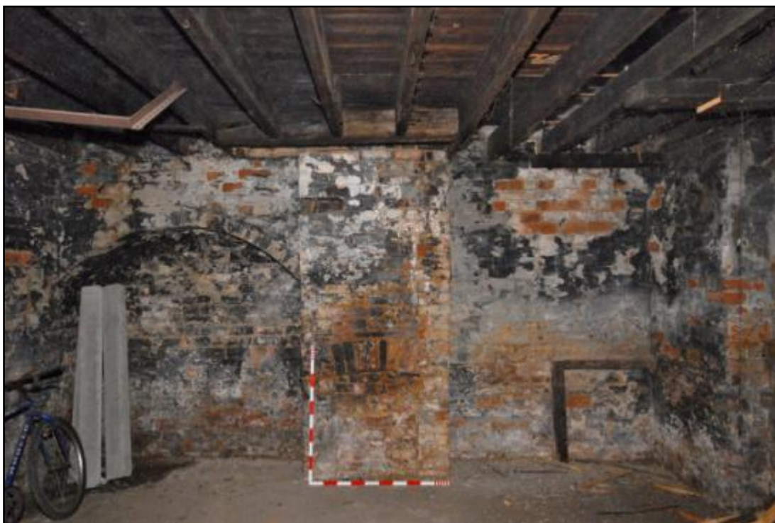
Building 1, ground floor, east wall with blocked fireplace flanked by arch Fig 26
