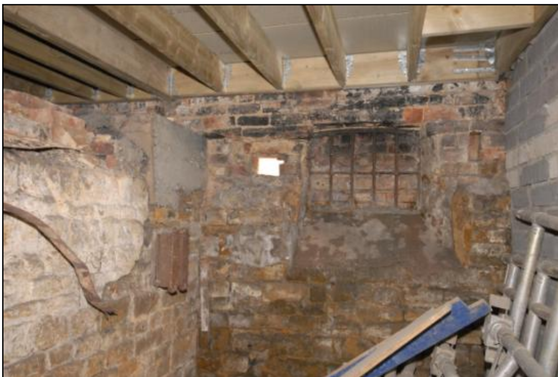
Room B2, blocked light well with electric box to the left Fig 56
