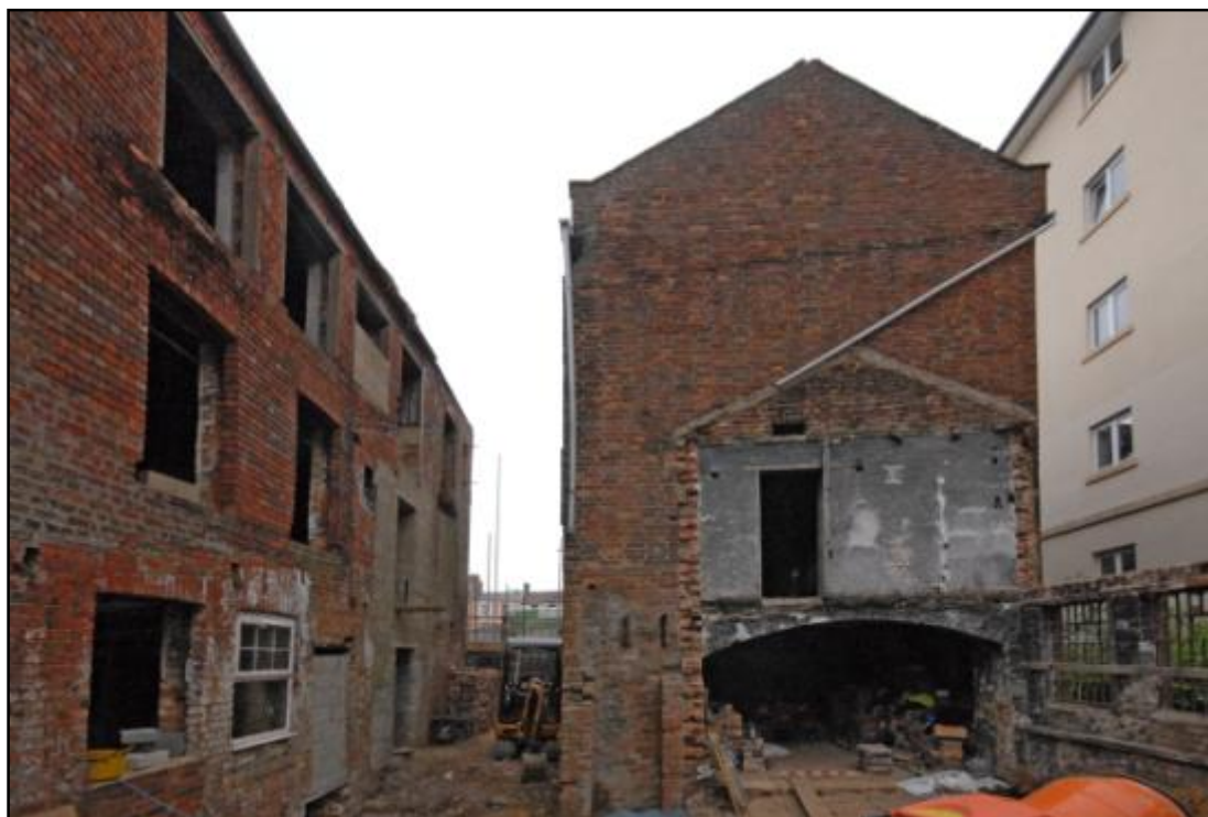
The west elevation of Building 1, showing scars of demolished annex, looking east Fig 16
