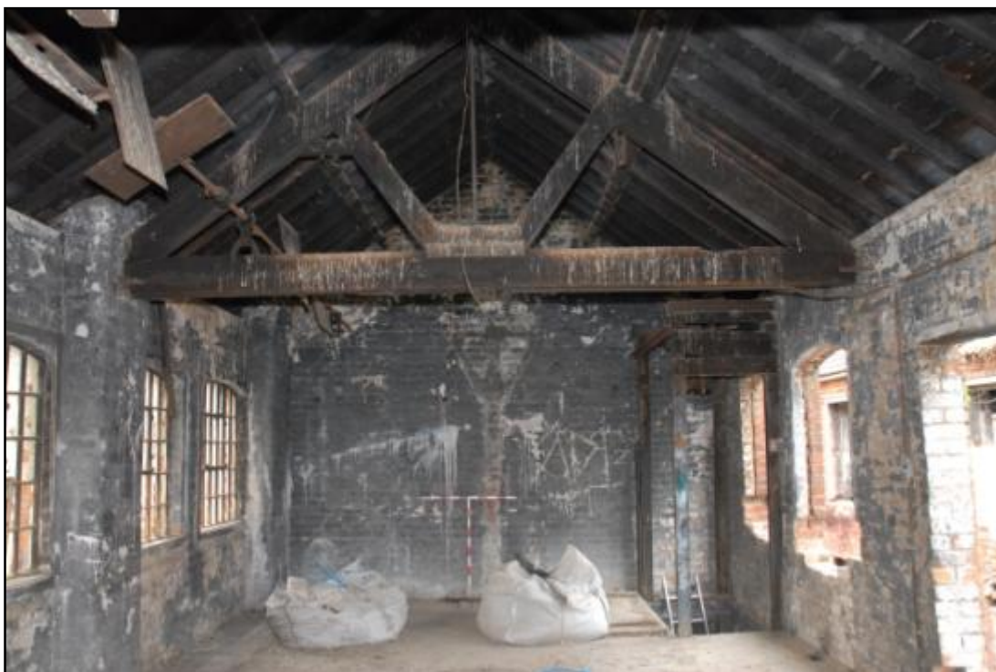
Building 1, second floor, looking east, showing lift shaft and scar of former machine support with drive shaft carried over the truss Fig 34
