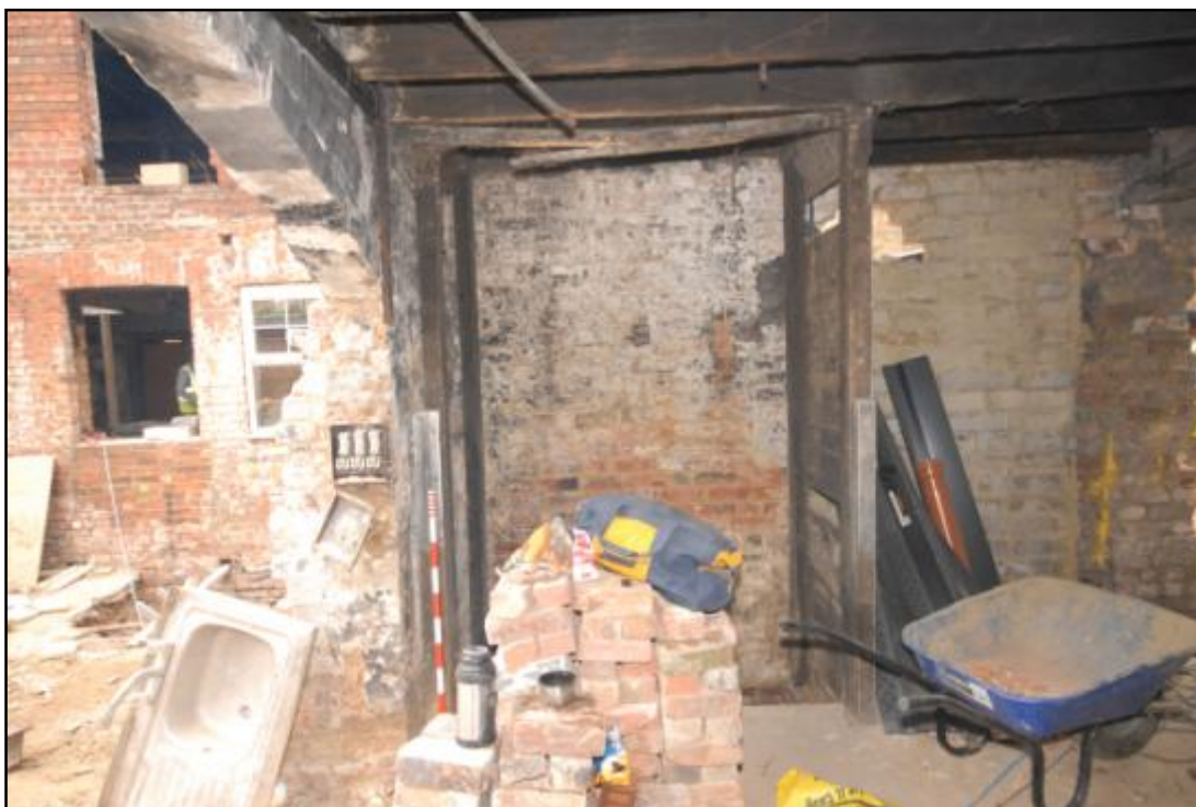
Building 1, ground floor, view of the lift shaft with electric box to the left Fig 30
