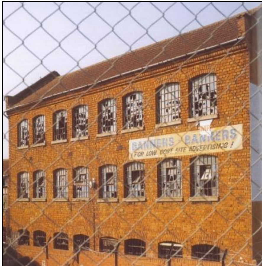
The south elevation of Building 1, prior to construction of new flats (Morrison, A, K & Bond, A, fig 54) Fig 13
