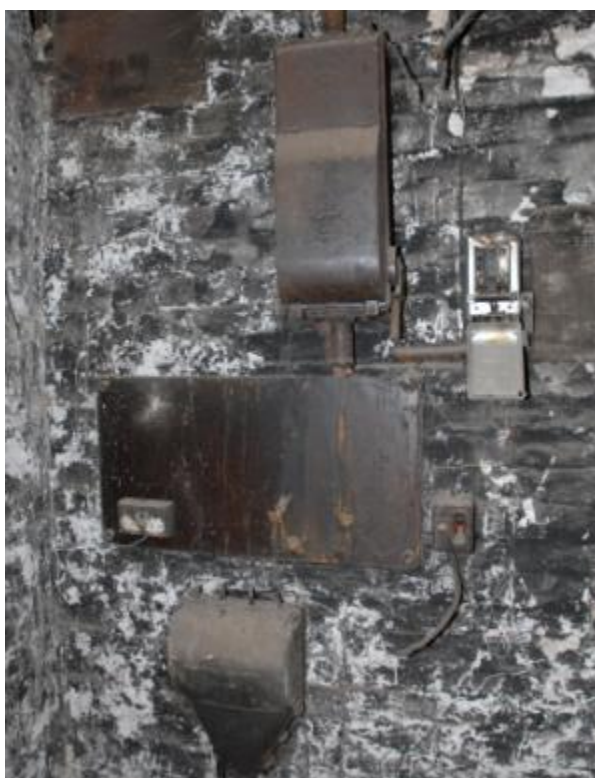
Detail of electric and utilities boxes in the lobby Fig 47
