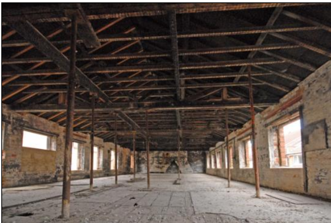
The second floor, looking west with chimney flues in the background Fig 65
