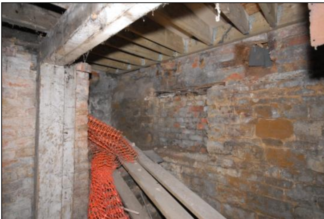
The blocked light well adjacent to the basement stair Fig 50
