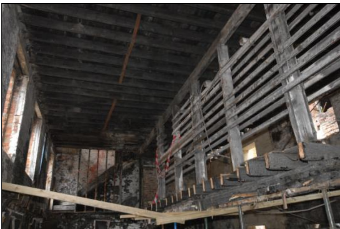
Building 2, the remains of the central first floor partition with the stairwell in the background, looking east Fig 64
