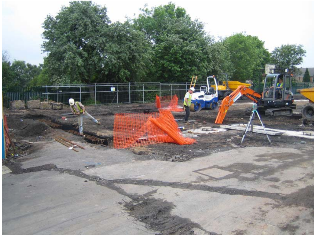
Plate 5: General view of watching brief area, note the square concrete base for temporary buildings centre right of photo, looking south-west
