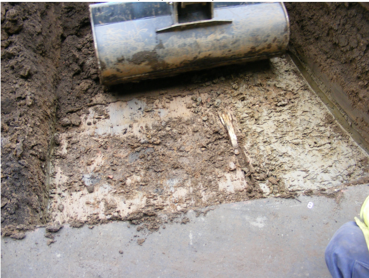
Fig 7: Excavation of the main trench, showing natural to right of picture and disturbed backfill of the sewer trench to left
