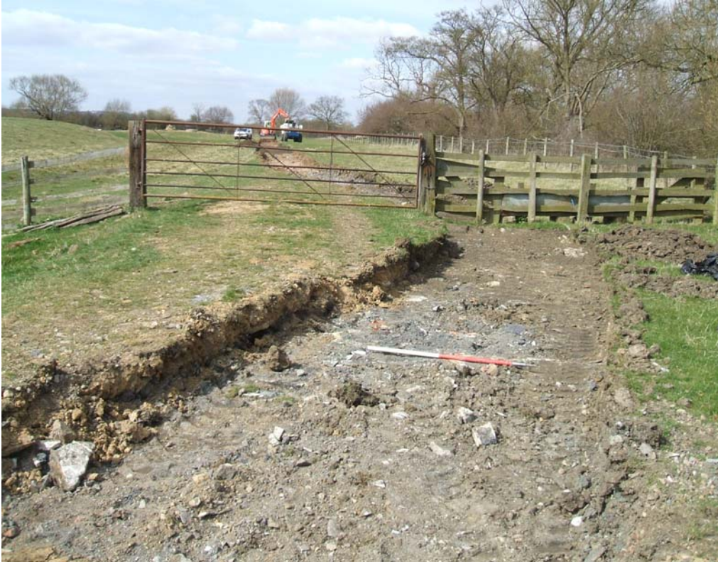
Fig 19: Diversion of footpath around a gate
