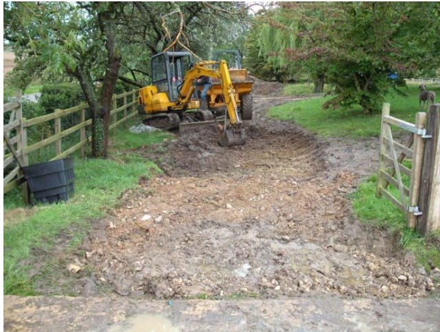
The access road being stripped, with an area of brick rubble in the middle of the frame, looking west Fig 9
