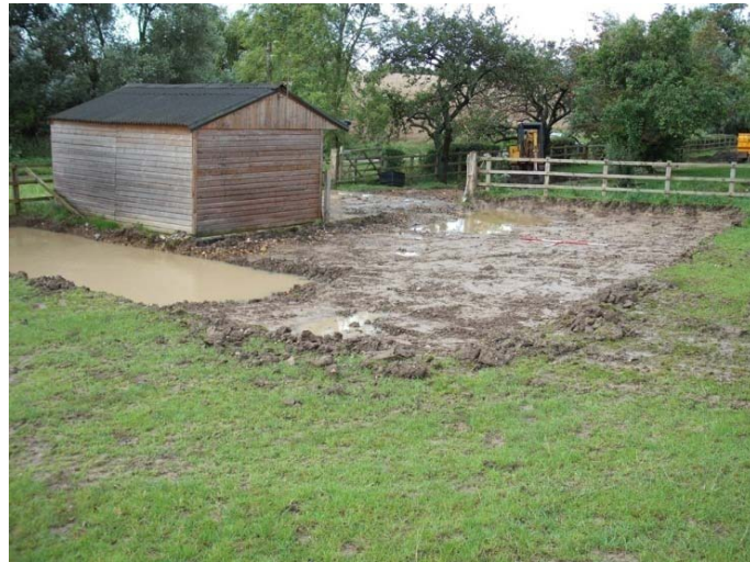
General view of the excavated area and the topsoil strip, looking south-west Fig 2
