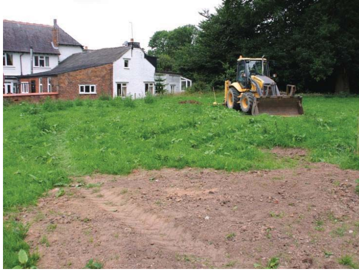
General view of the site prior to excavation, looking south-west towards Bargates Cottage and The Gables Fig 3
