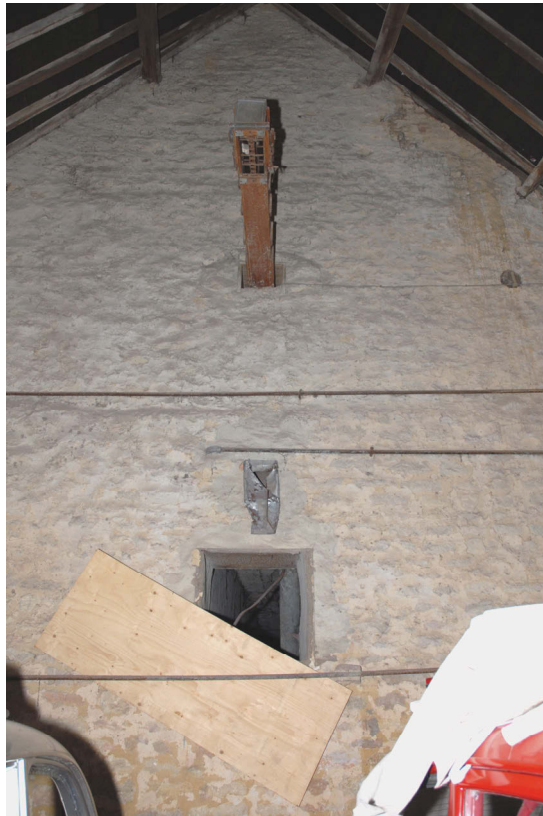
The tie rod and surviving machinery and openings in the south-west wall of Barn 1
