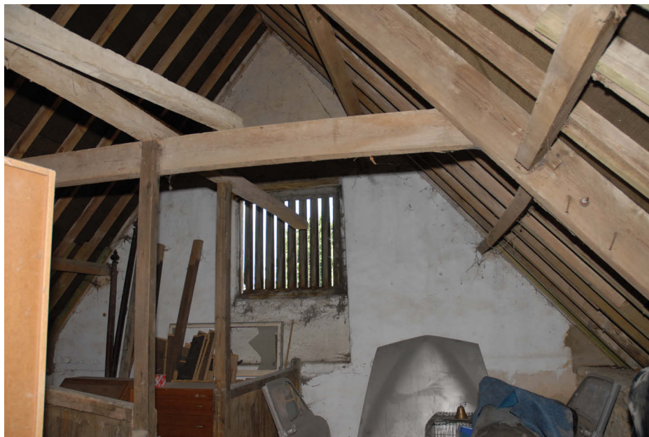
The partially blocked window in the north-west wall of the hayloft Fig 18
