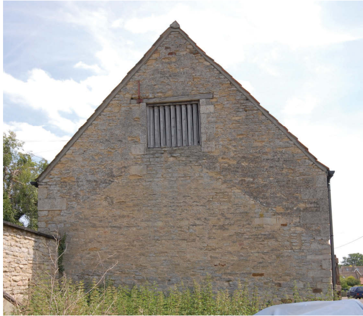
Scarring from the cattle byres on the north-west wall of the Store and Hayloft above Fig 19
