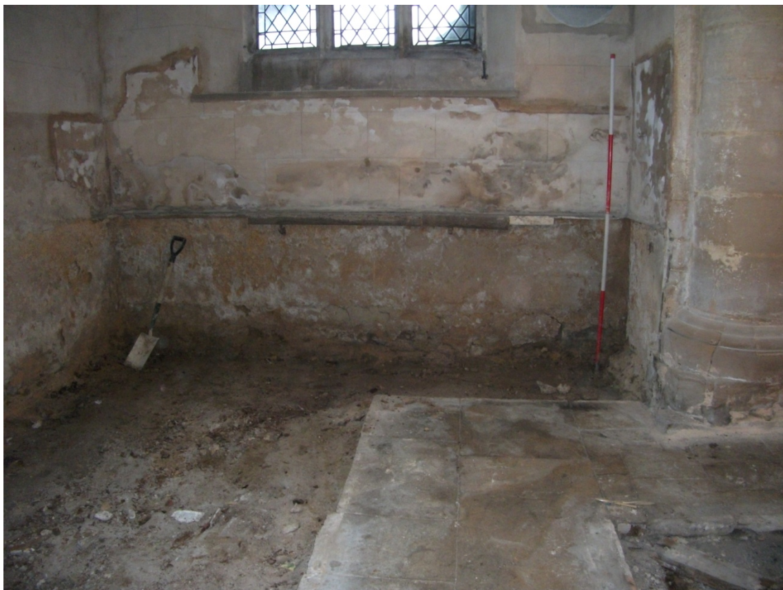
The west wall of the south aisle after removal of the timber cladding Fig 7
