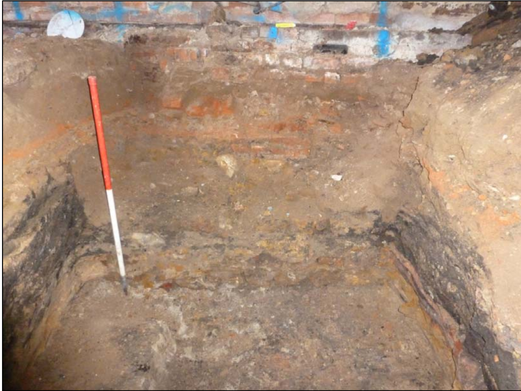
Wall exposed in the temporary works excavation in room G1, 5 Sheep Street Fig 17
