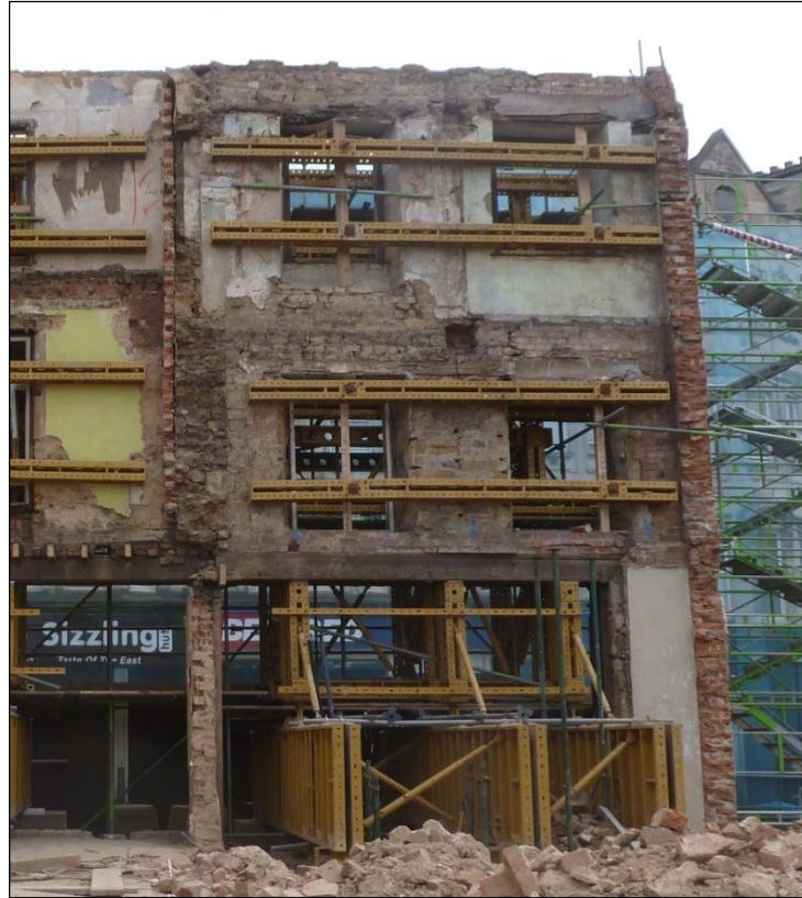
The internal facade of 5 Sheep Street, showing the rebuilt southern part with concrete window lintels Fig 14
