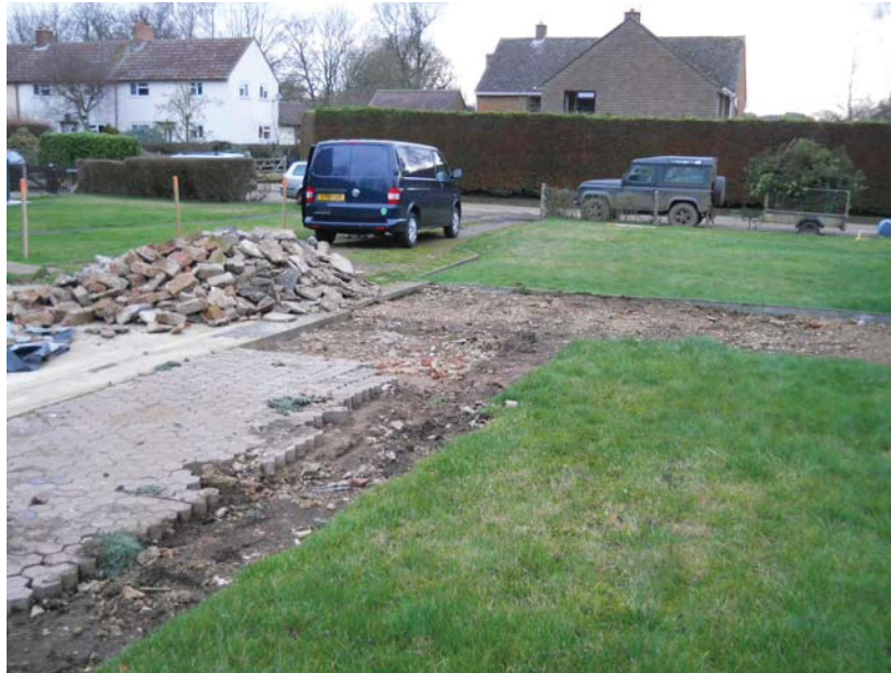
The site, with the demolished garage in the foreground, looking north Fig 2
