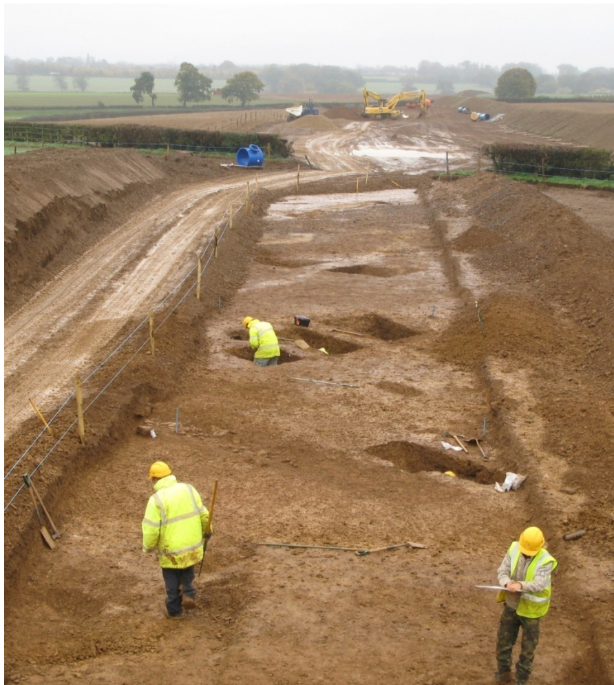
General view of Roman ditches at White Hill Lodge, looking south Fig 5.13
