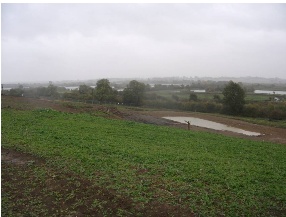
Plate 2: General view of one of the balancing ponds, viewed to the north-east
