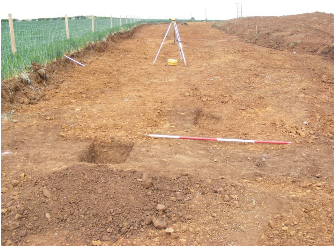
Plate 3: General view of the features in the south-west corner of the site
