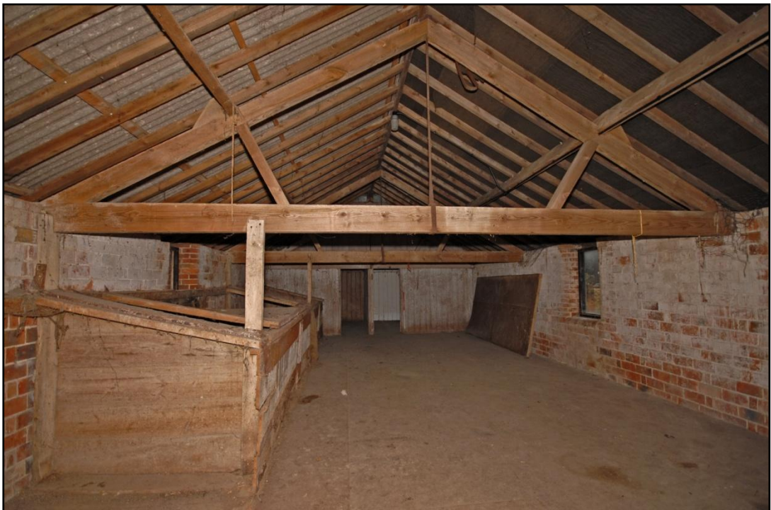
The first floor, looking west, showing surviving chicken coops and roof structure Fig 18
