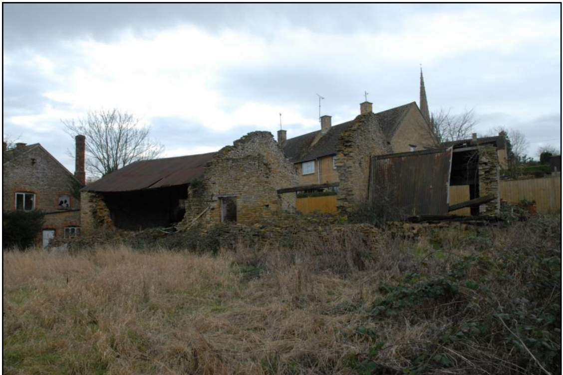
General view of the site prior to demolition of the outbuildings, looking south-east Fig 21
