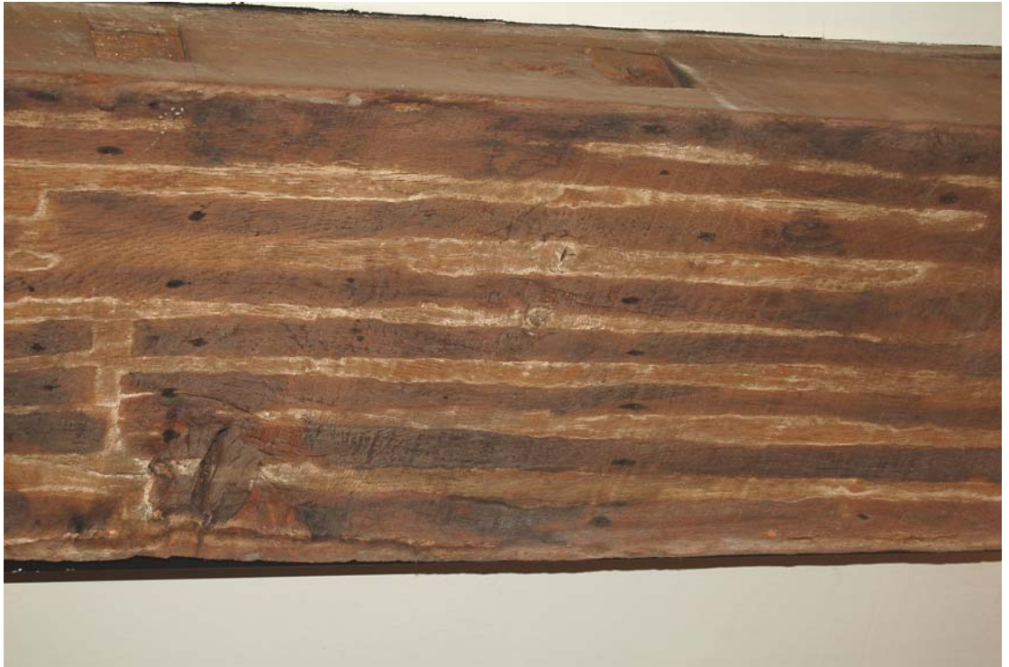
Fig 13: First floor, close up of underside of beam showing scar of lath and plaster ceiling
