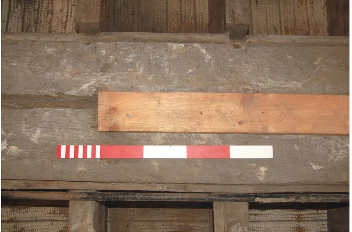
Fig 9: First floor partition slot in beam C
