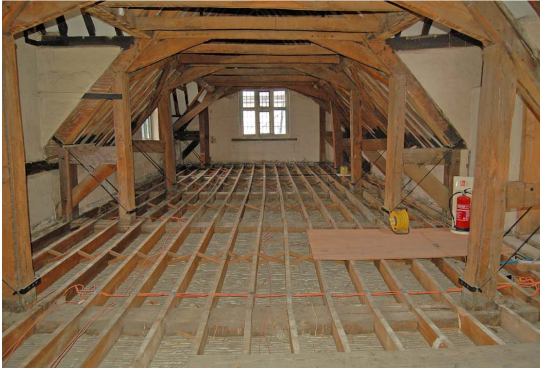
Fig 20: General view of the attic floorboards removed, showing the modern joists and original beams
